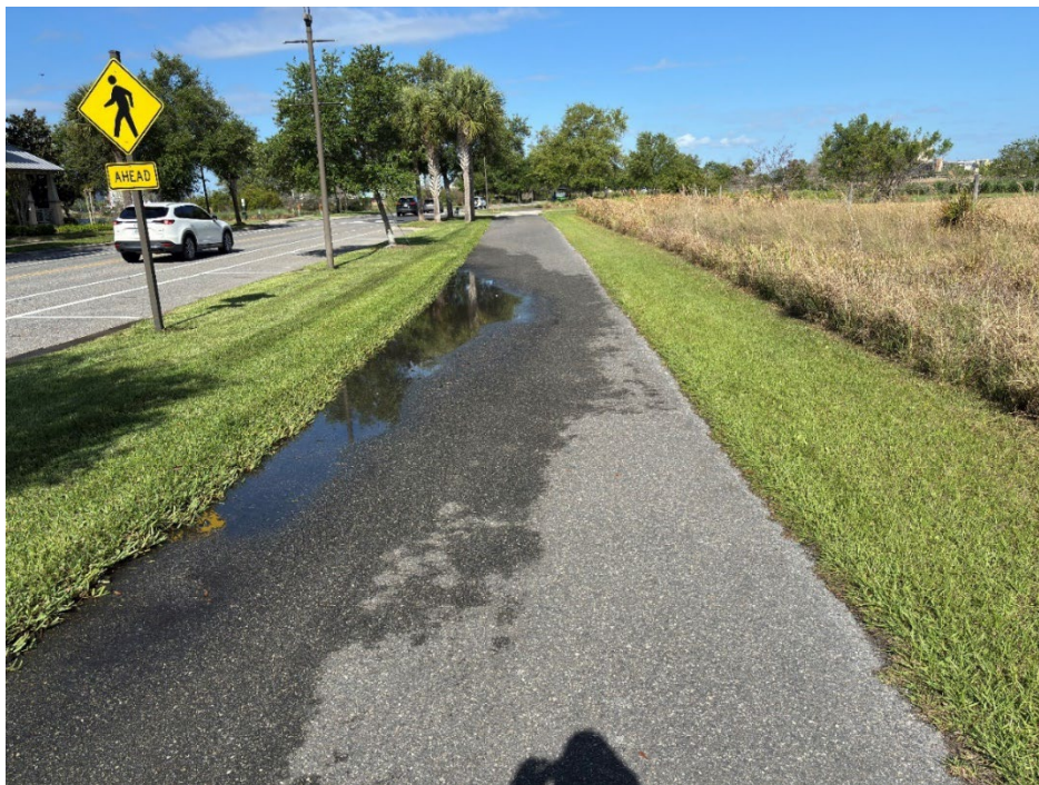
Photo 33.1 – Water Ponding (New Photo – 2026 Assessment)
