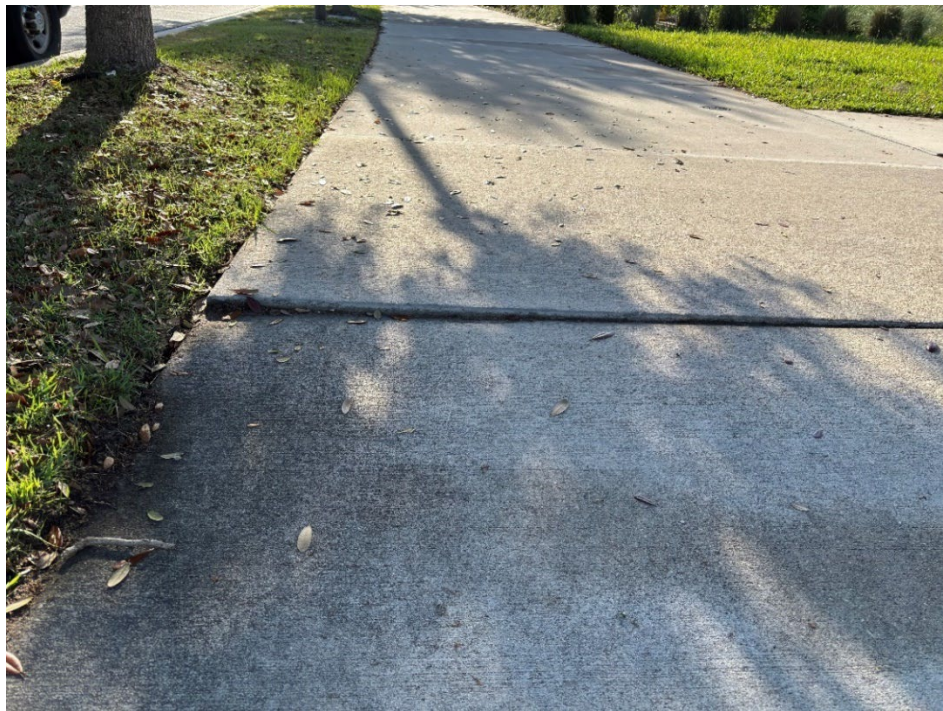
Photo 15.1 – Concrete Slab Movement (New Photo – 2026 Assessment)
