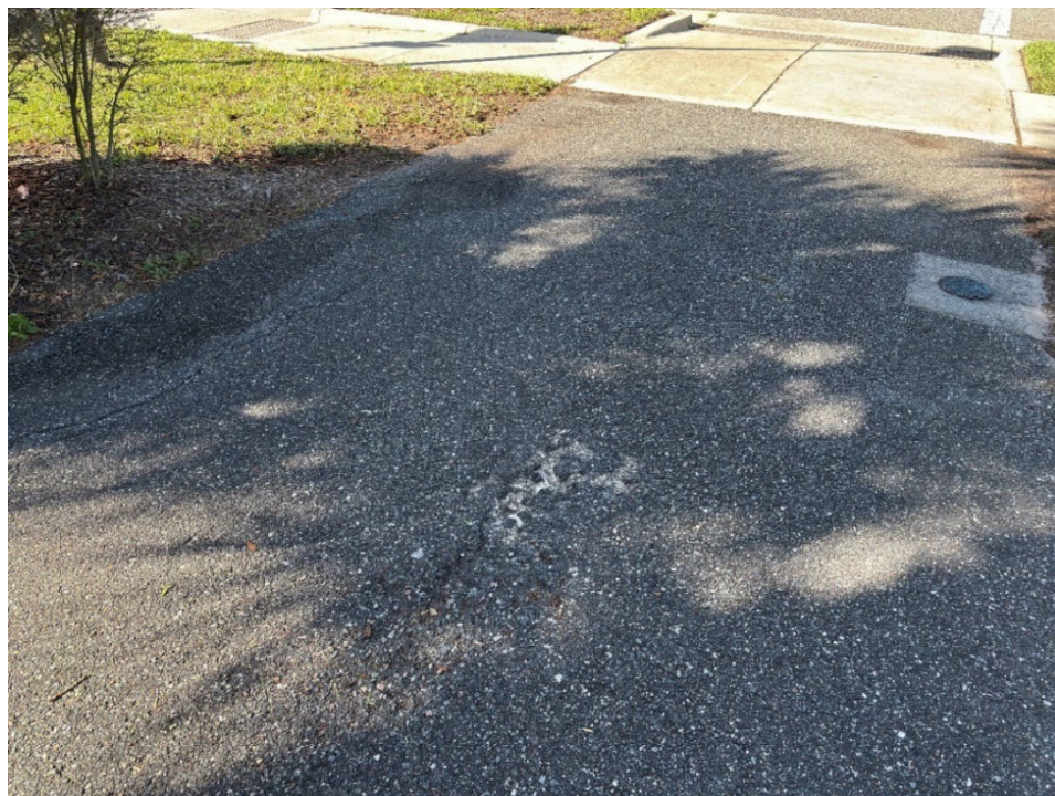
Photo 25.1 – Asphalt Damage (New Photo – 2026 Assessment)
