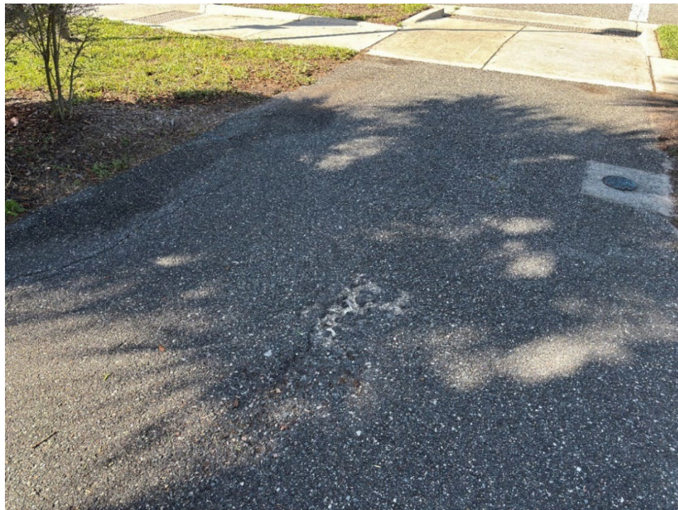
Photo 25.1 – Asphalt Damage (New Photo – 2026 Assessment)
