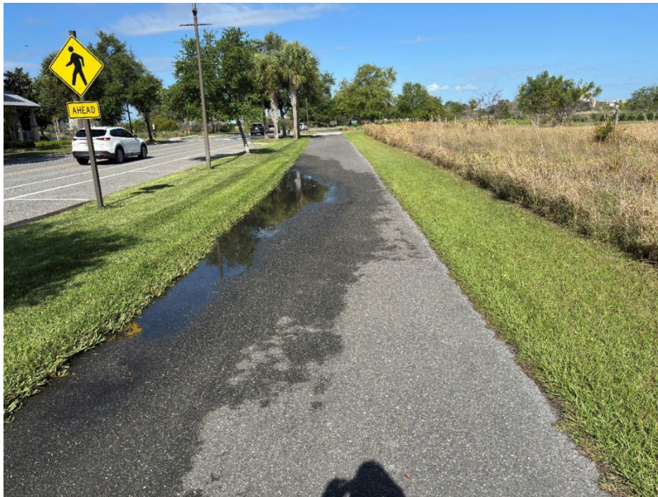
Photo 33.1 – Water Ponding (New Photo – 2026 Assessment)
