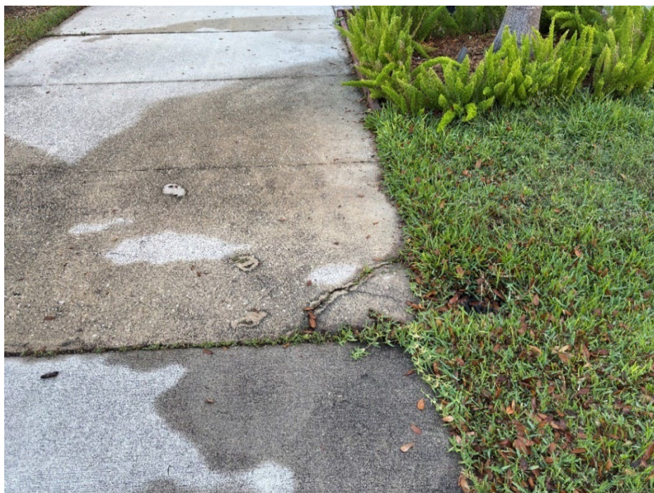
Photo 11 Cracked Concrete and Base Failure at Yard Drain (Base Failure Progressing) (Refer to Prior Photo 15 – 2025 Assessment)
