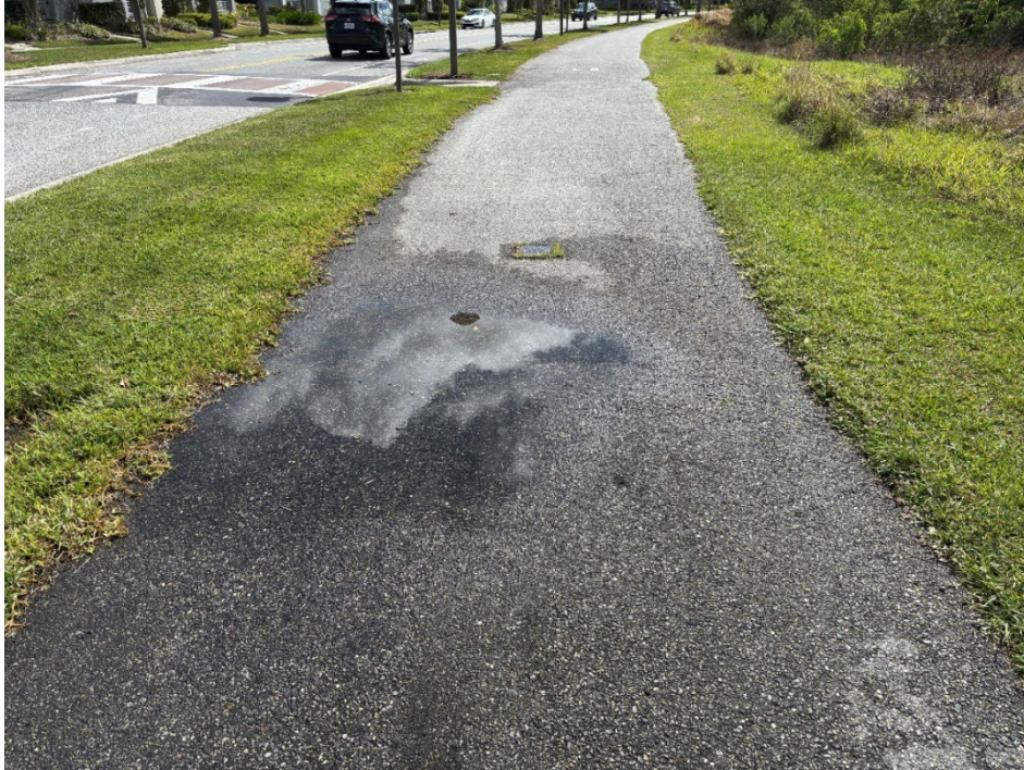
Photo 42.3 – Water Ponding (New Photo – 2026 Assessment)
