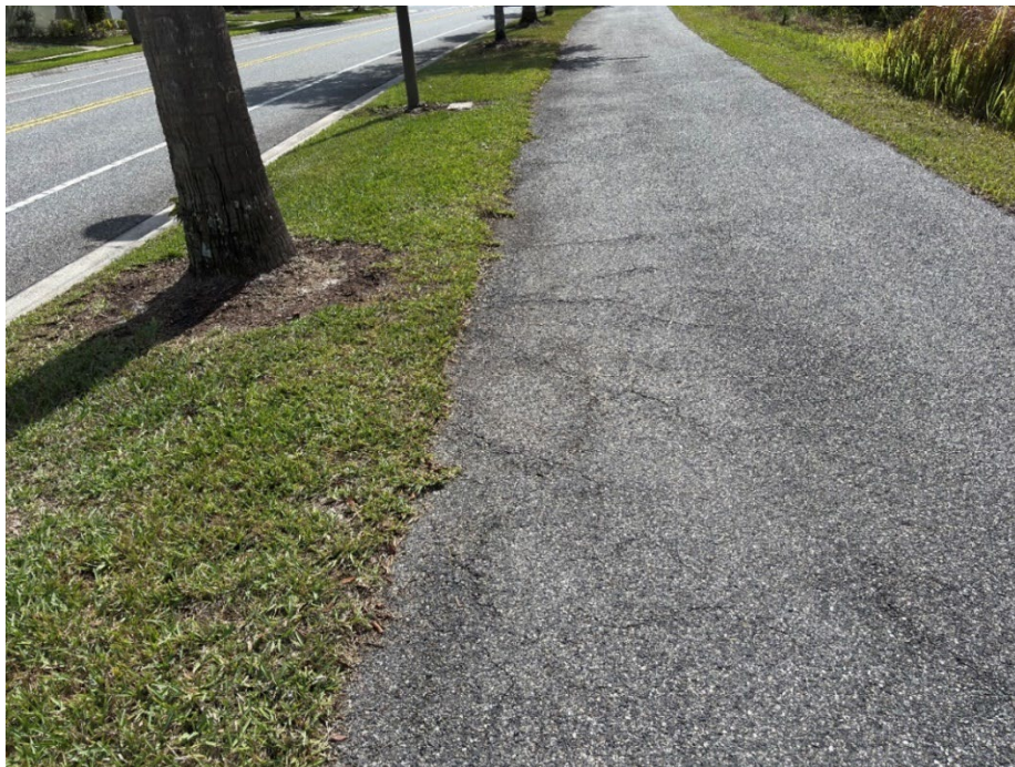
Photo 43 - Asphalt Raveling and Base Failure (No Observed Changes) (Refer to Prior Photo 58 – 2025 Assessment)
