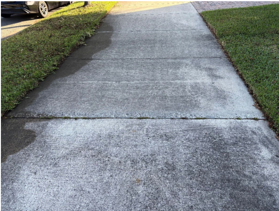
Photo 9 – Concrete Slab Movement (Previously Ground Down - Additional Ponding Area Observed) (Refer to Prior Photo 11 – 2025 Assessment)
