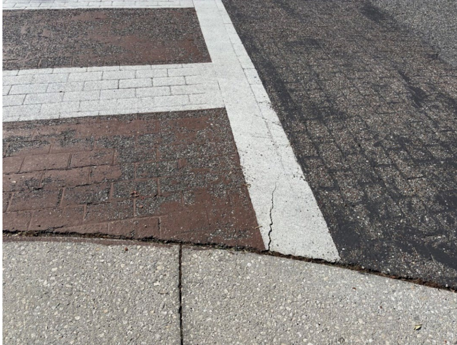
Photo 27 Deteriorating Thermoplastic and Worn Crosswalk Coloration (No Observed Changes) (Refer to Prior Photo 36 – 2025 Assessment)
