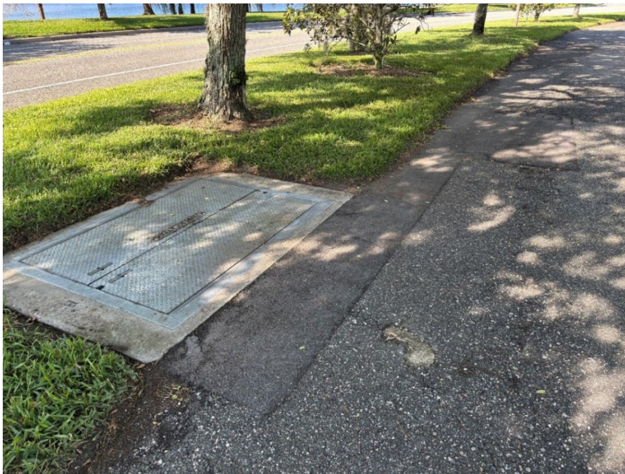
Photo 28 Poor Quality Asphalt Patch (No Observed Changes) (Refer to Prior Photo 37 – 2025 Assessment)
