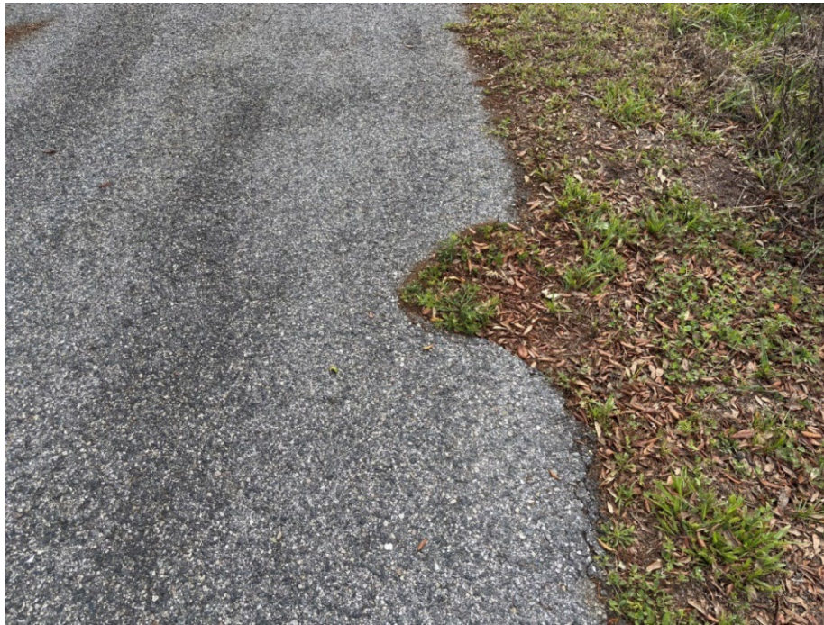
Photo 48 - Asphalt Edge Failure (No Observed Changes) (Refer to Prior Photo 66 – 2025 Assessment)
