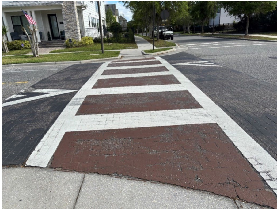
Photo 38 Deteriorating Thermoplastic and Worn Crosswalk Coloration (No Observed Changes) (Refer to Prior Photo 53 – 2025 Assessment)
