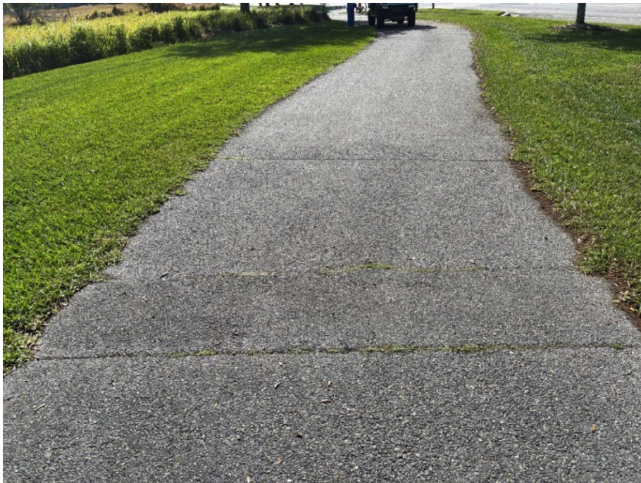
Photo 34 - Cracked Asphalt and Asphalt Raveling (No Observed Changes) (Refer to Prior Photo 47 – 2025 Assessment)
