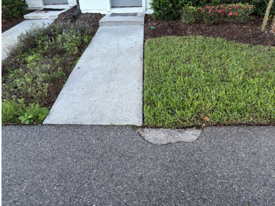
Photo 7 - Poor Asphalt Patch (No Observed Changes) (Refer to Prior Photo 8 – 2025 Assessment)
