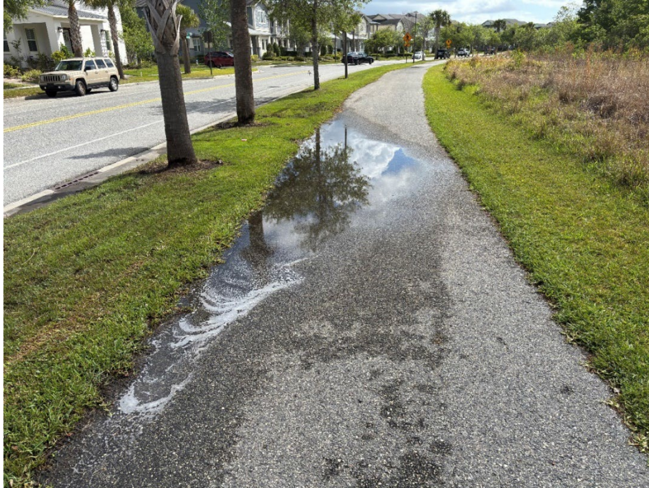
Photo 42.1 – Water Ponding (New Photo – 2026 Assessment)
