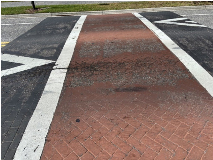
Photo 46 Deteriorating Thermoplastic, Worn Crosswalk Coloration, and Asphalt Deformation (Further Deterioration Observed) (Refer to Prior Photo 62 – 2025 Assessment)
