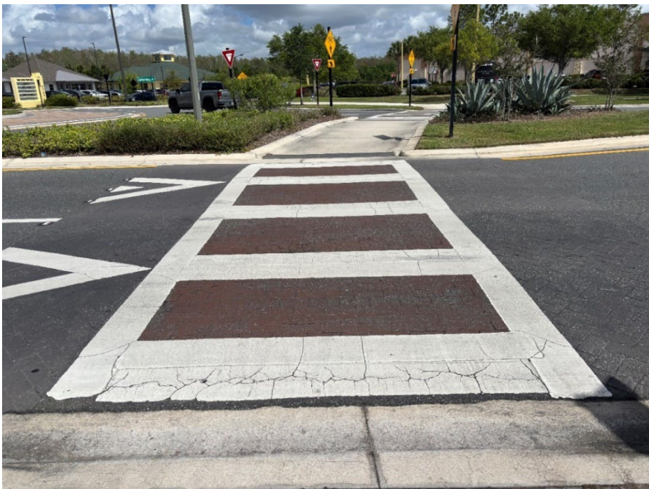
Photo 54 Deteriorating Thermoplastic and Worn Crosswalk Coloration (No Observed Changes) (Refer to Prior Photo 74 – 2025 Assessment)
