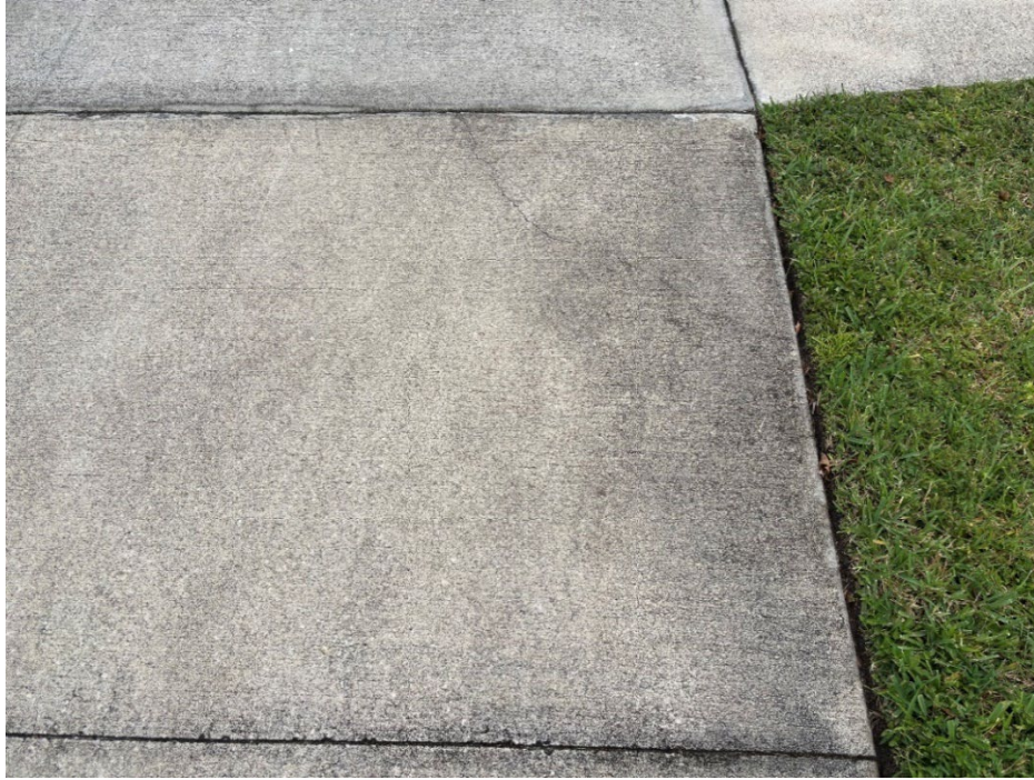
Photo 10 - Cracked Concrete and Base Failure (No Observed Changes) (Refer to Prior Photo 14 – 2025 Assessment)
