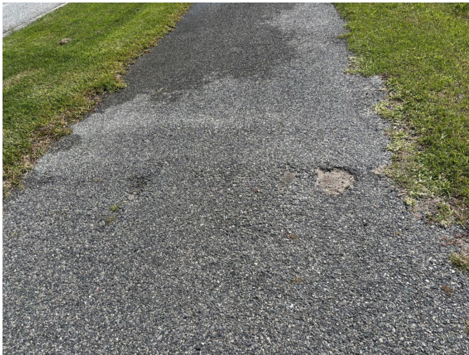
Photo 42.2 – Asphalt Spalling (New Photo – 2026 Assessment)
