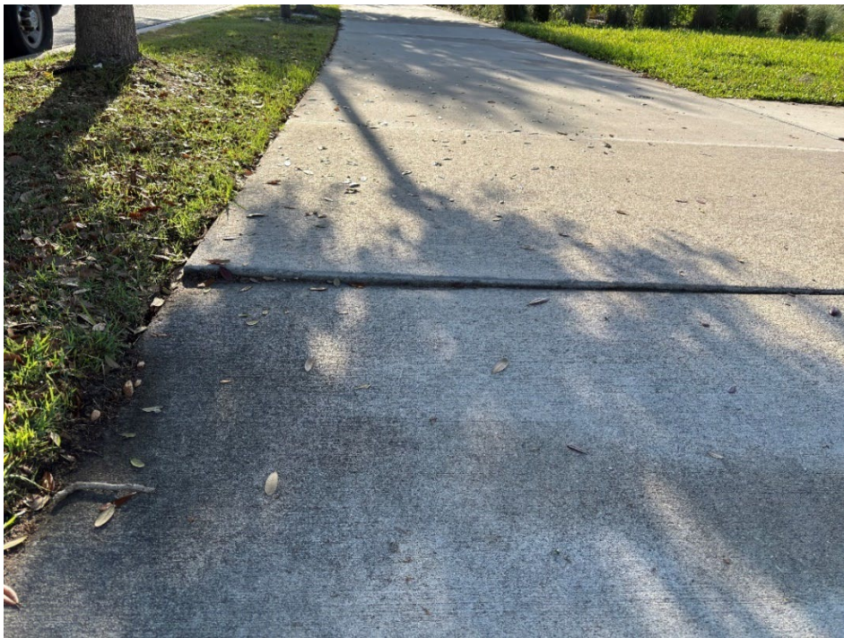
Photo 15.1 – Concrete Slab Movement (New Photo – 2026 Assessment)
