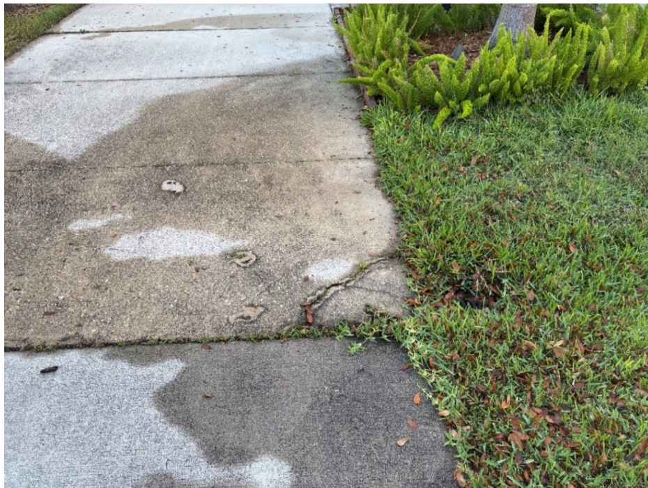
Photo 11 Cracked Concrete and Base Failure at Yard Drain (Base Failure Progressing) (Refer to Prior Photo 15 – 2025 Assessment)
