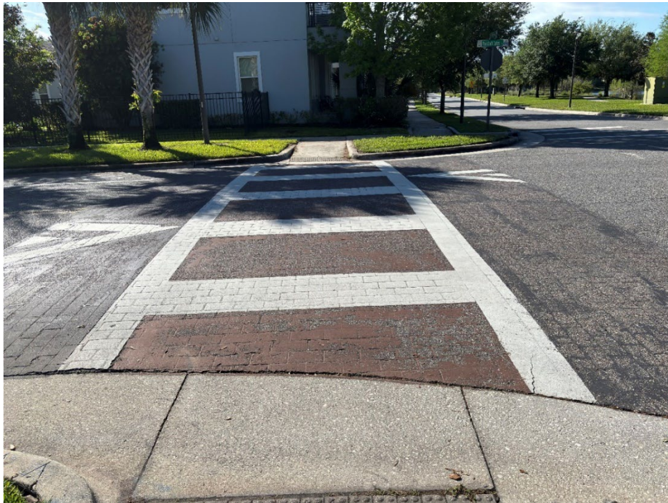
Photo 26 Deteriorating Thermoplastic and Worn Crosswalk Coloration (No Observed Changes) (Refer to Prior Photo 35 – 2025 Assessment)
