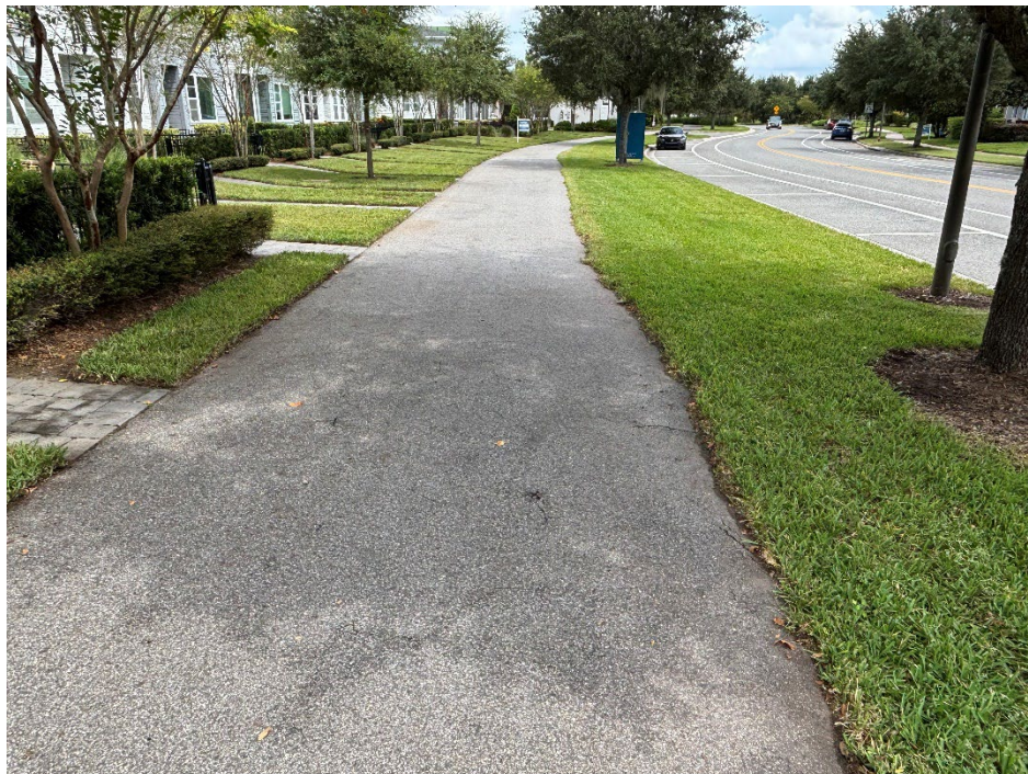
Photo 30 - Asphalt Edge Failure (No Observed Changes) (Refer to Prior Photo 39 – 2025 Assessment)
