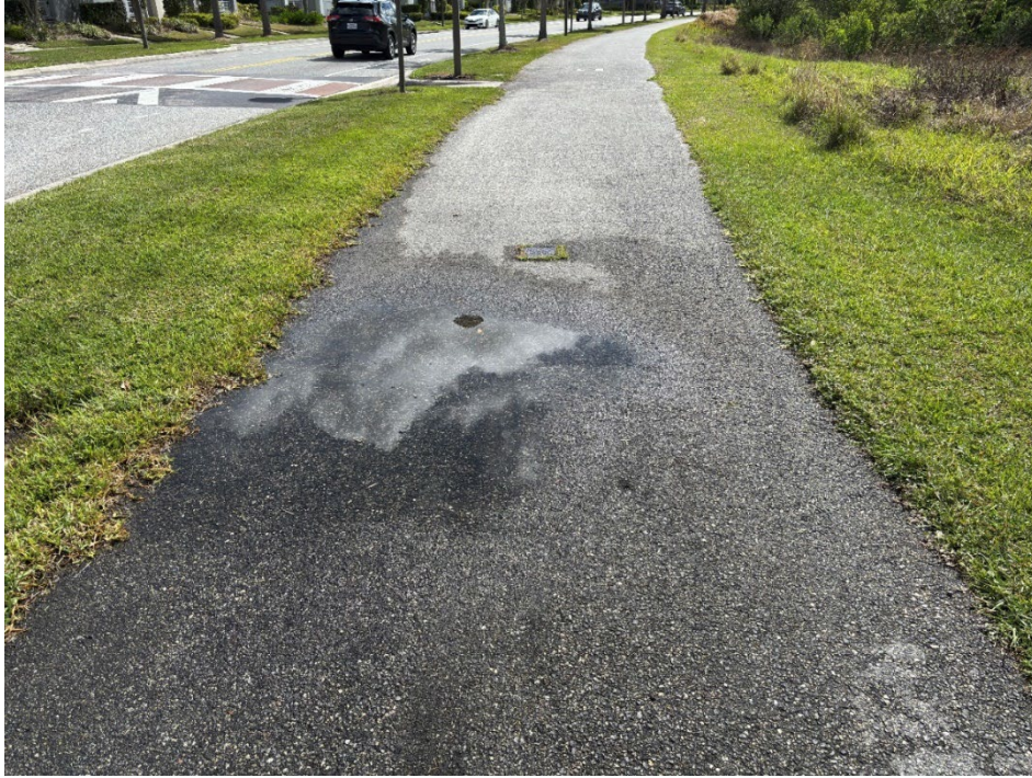
Photo 42.3 – Water Ponding (New Photo – 2026 Assessment)
