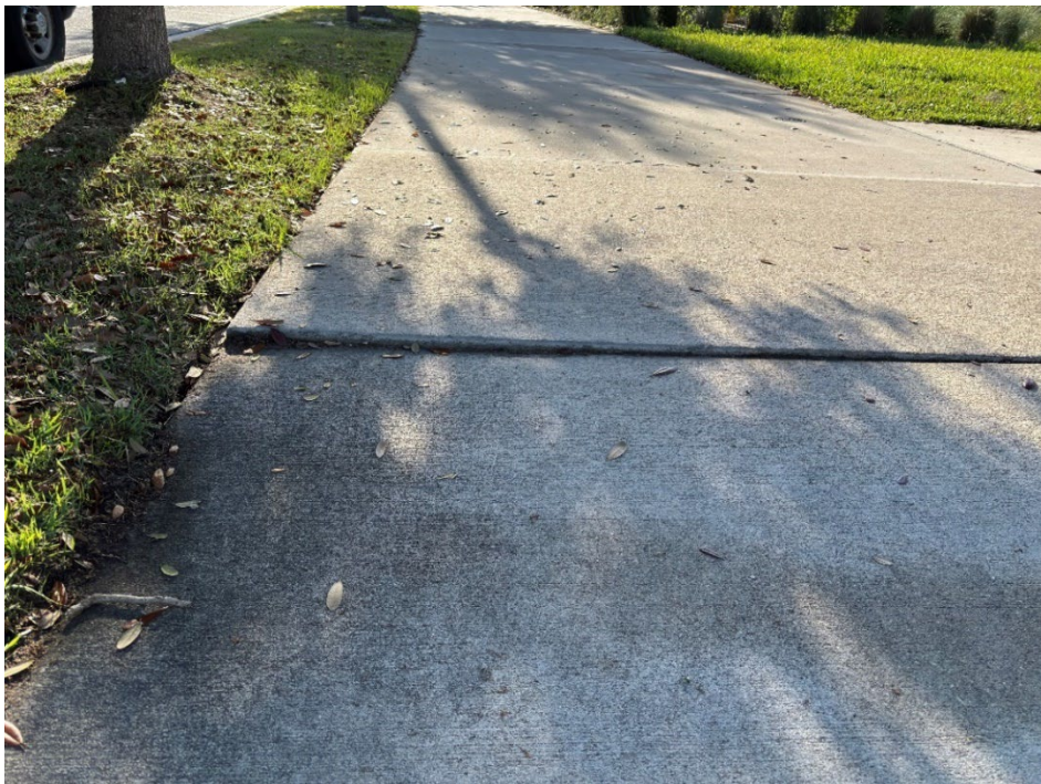
Photo 15.1 – Concrete Slab Movement (New Photo – 2026 Assessment)
