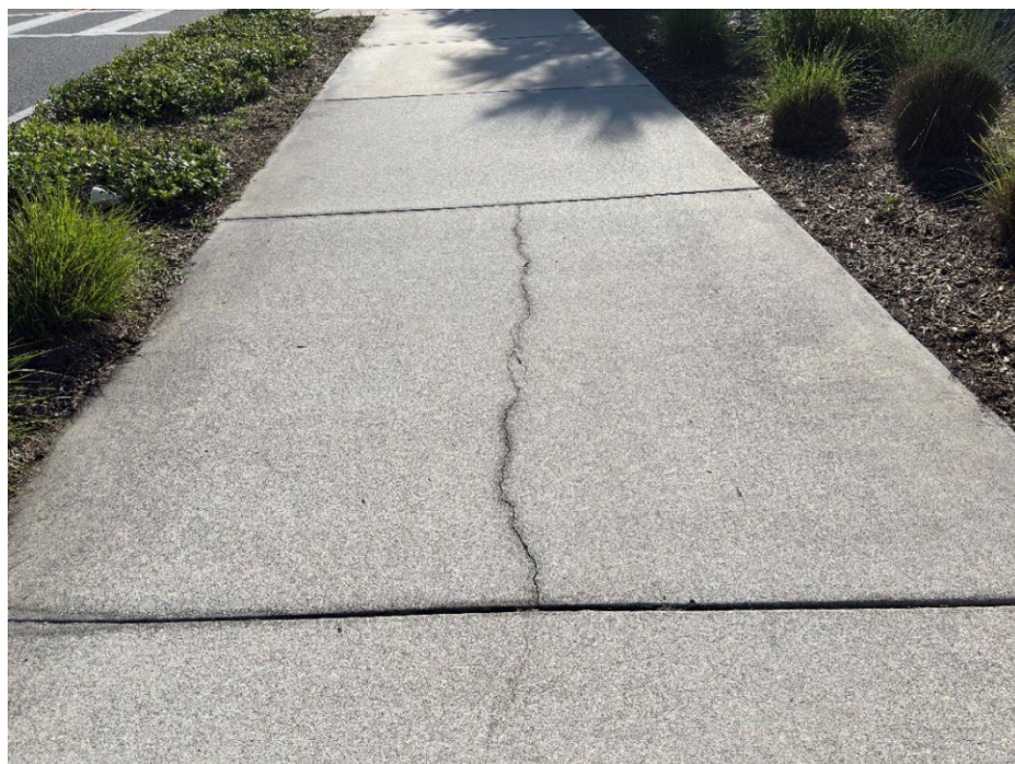
Photo 19 - Cracked Concrete (No Observed Changes) (Refer to Prior Photo 24 – 2025 Assessment)
