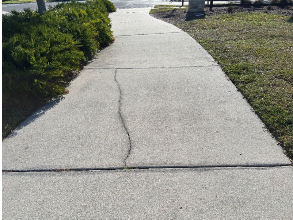
Photo 16 - Cracked Concrete (No Observed Changes) (Refer to Prior Photo 21 – 2025 Assessment)
