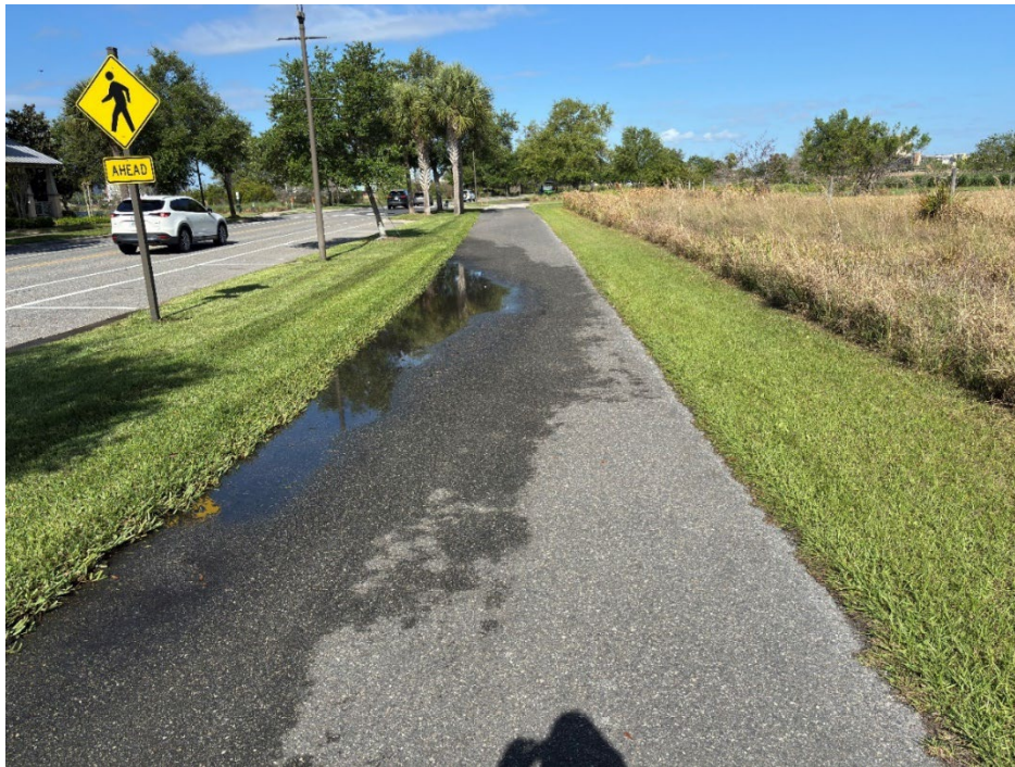
Photo 33.1 – Water Ponding (New Photo – 2026 Assessment)
