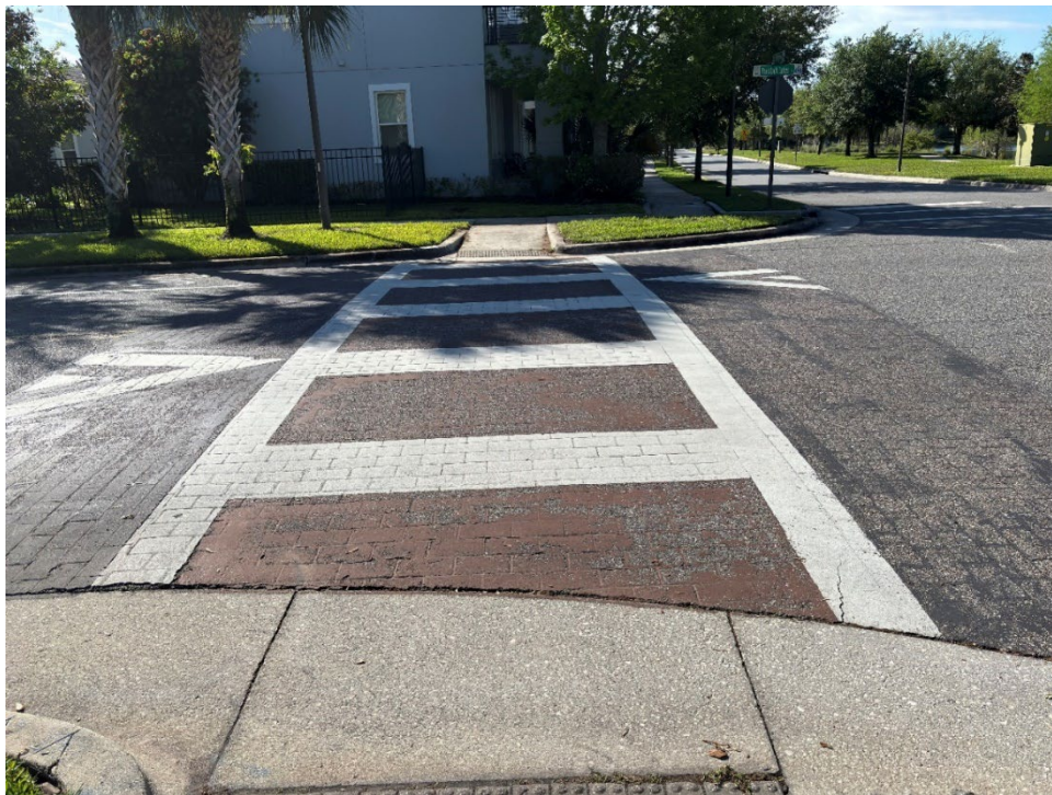
Photo 26 Deteriorating Thermoplastic and Worn Crosswalk Coloration (No Observed Changes) (Refer to Prior Photo 35 – 2025 Assessment)
