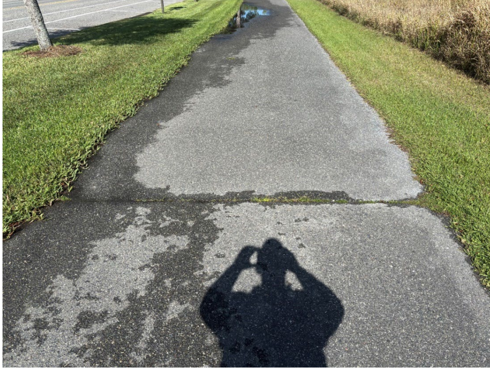
Photo 33 Cracked Asphalt from Side to Side (Increased Cracking Severity Observed) (Refer to Prior Photo 43 – 2025 Assessment)
