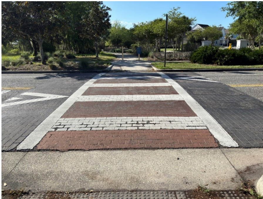
Photo 22 - Deteriorating Thermoplastic and Worn Crosswalk Coloration (Further Deterioration Observed) (Refer to Prior Photo 30 – 2025 Assessment)
