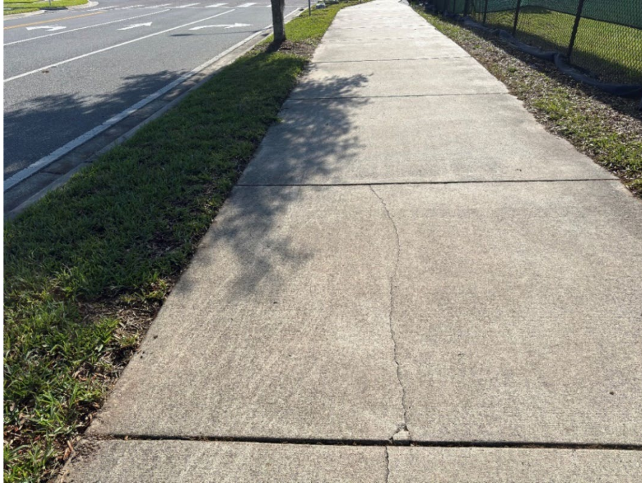
Photo 21 - Surficial Cracked Concrete (No Observed Changes) (Refer to Prior Photo 29 – 2025 Assessment)
