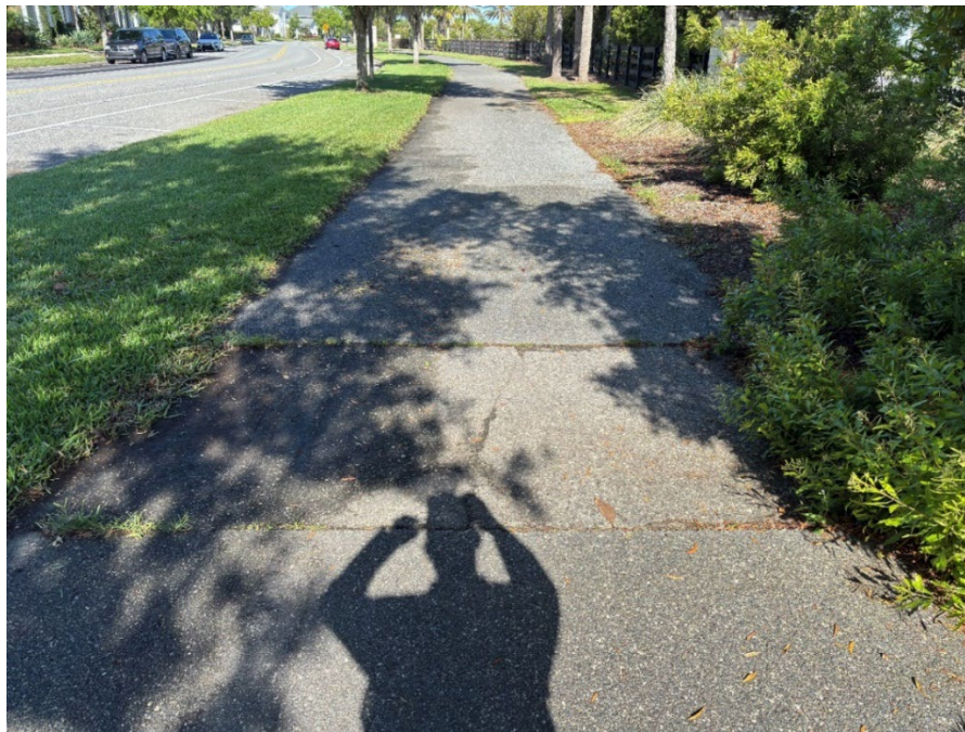
Photo 24 Poor Quality Asphalt Patch (Asphalt Patch Edge Failure Observed) (Refer to Prior Photo 33 – 2025 Assessment)
