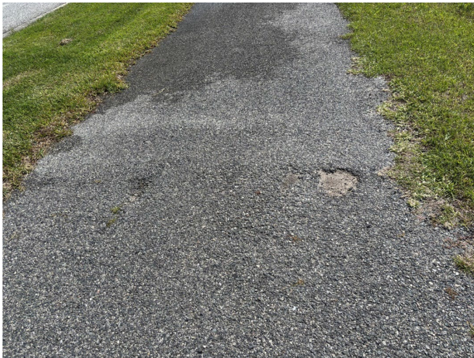
Photo 42.2 – Asphalt Spalling (New Photo – 2026 Assessment)
