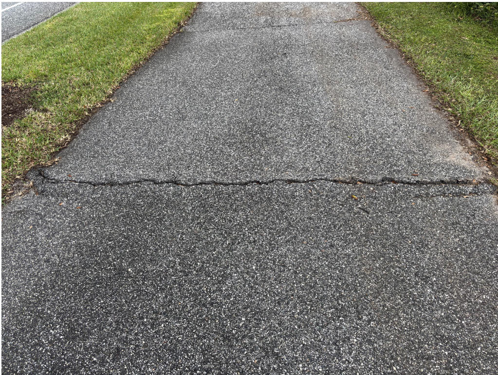
Photo 64 – Asphalt Patch Lifting
