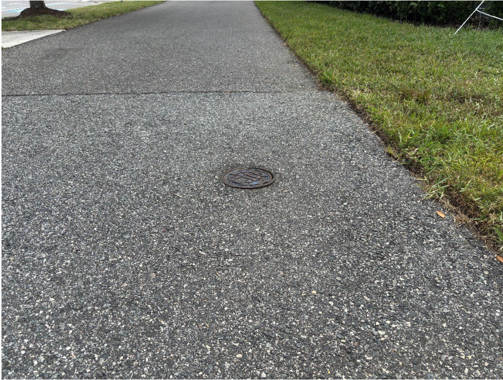
Photo 9 – Valve Cover Approximately 1/2-inch Reveal
