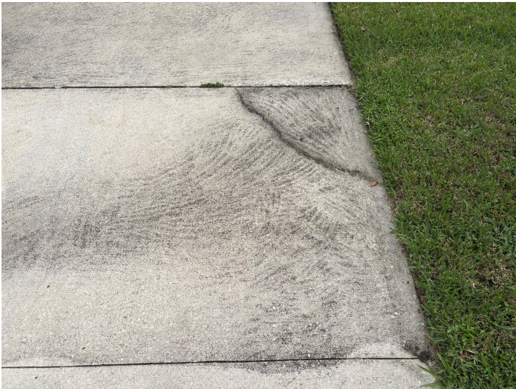
Photo 16 – Cracked Concrete and Base Failure
