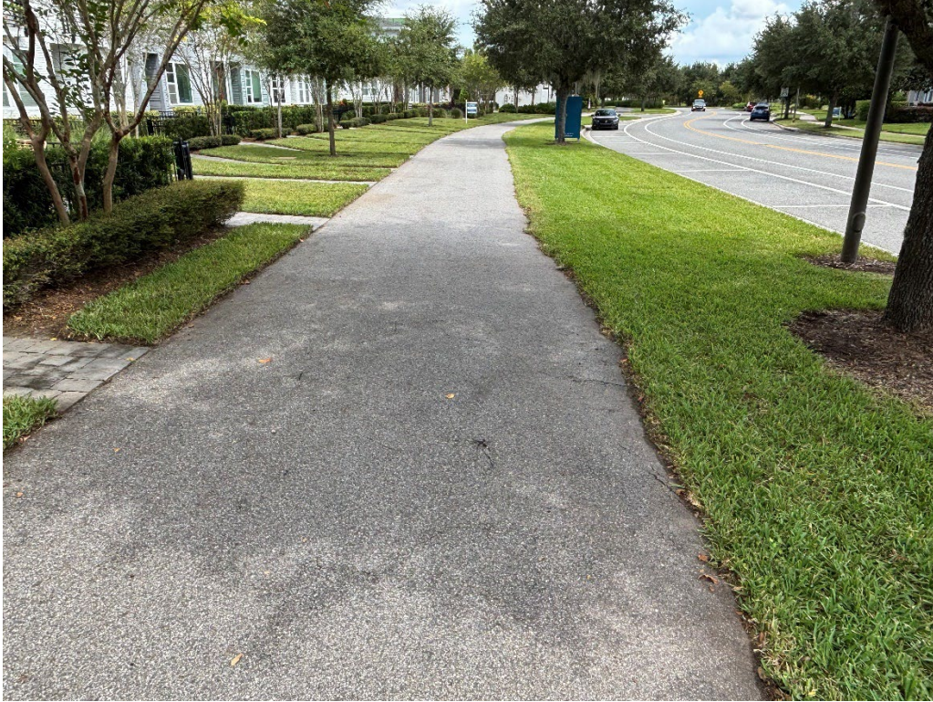
Photo 39 – Asphalt Edge Failure
