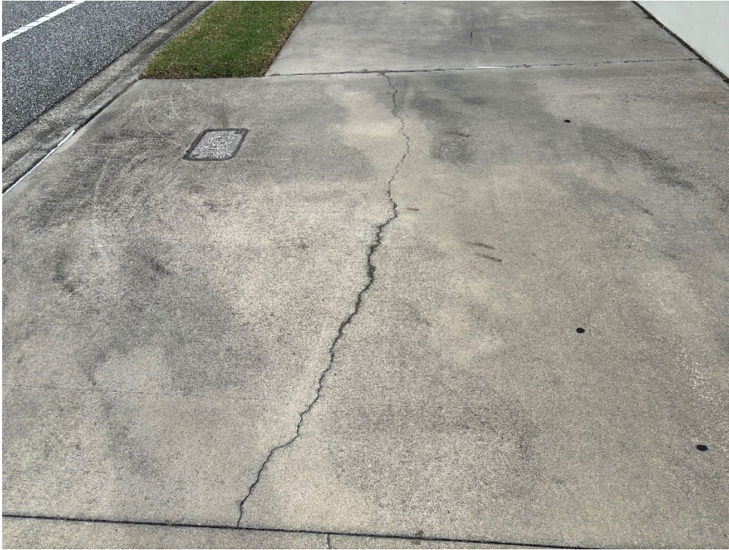
Photo 71 – Surficial Cracked Concrete
