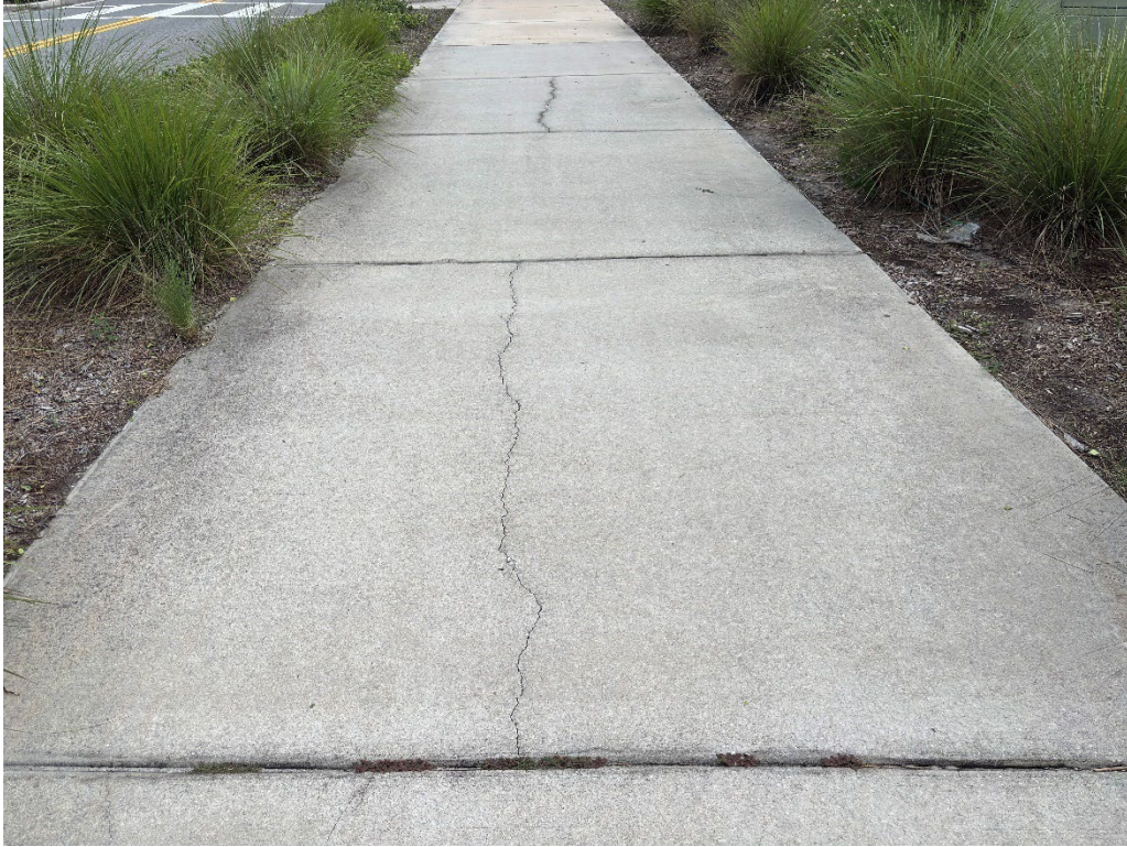
Photo 23 – Surficial Cracked Concrete
