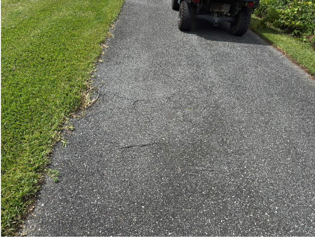
Photo 31 – Asphalt Raveling and Base Failure
