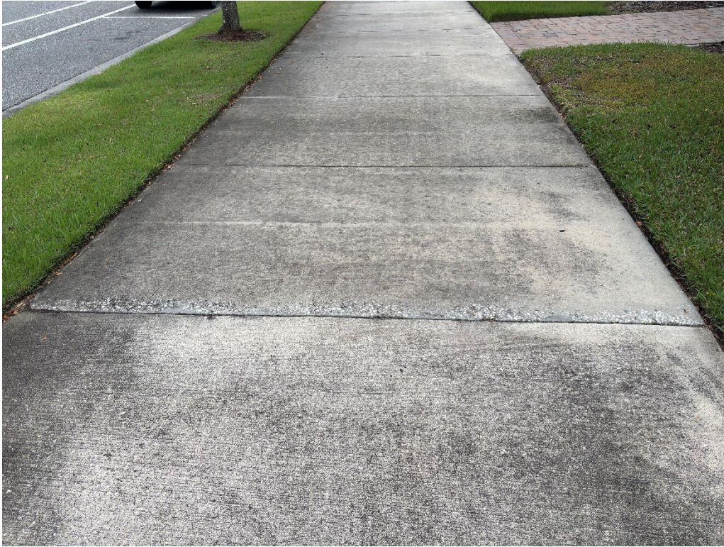
Photo 11 – Concrete Slab Movement (Previously Ground Down)
