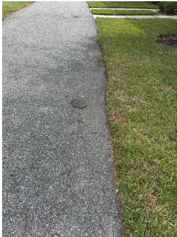
Photo 2 – Asphalt Pavement Edge Failure
