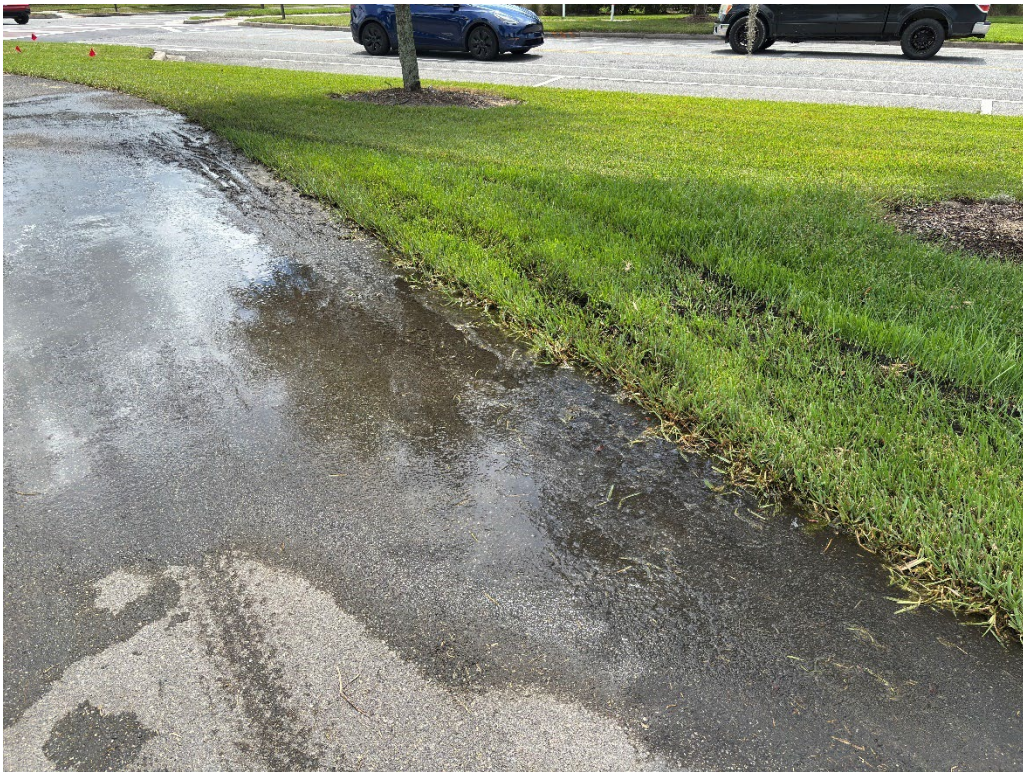
Photo 46 – Asphalt Raveling in Low Area
