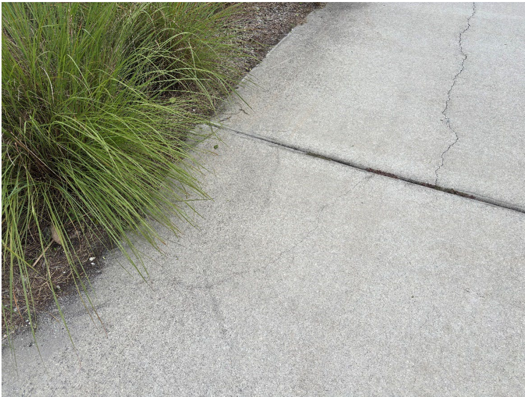
Photo 22 – Surficial Cracked Concrete
