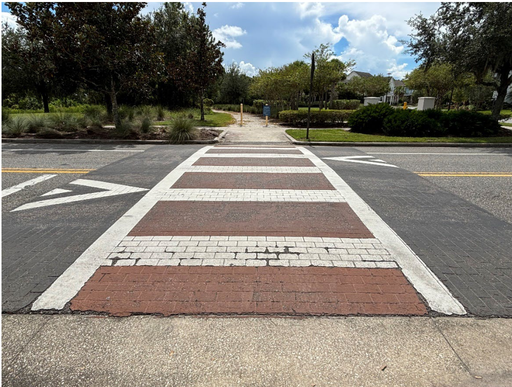
Photo 30 - Deteriorating Thermoplastic and Worn Crosswalk Coloration
