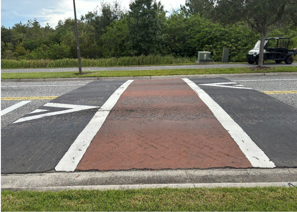
Photo 61 – Deteriorating Thermoplastic, Worn Crosswalk Coloration, and Asphalt Speed Table Deformation
