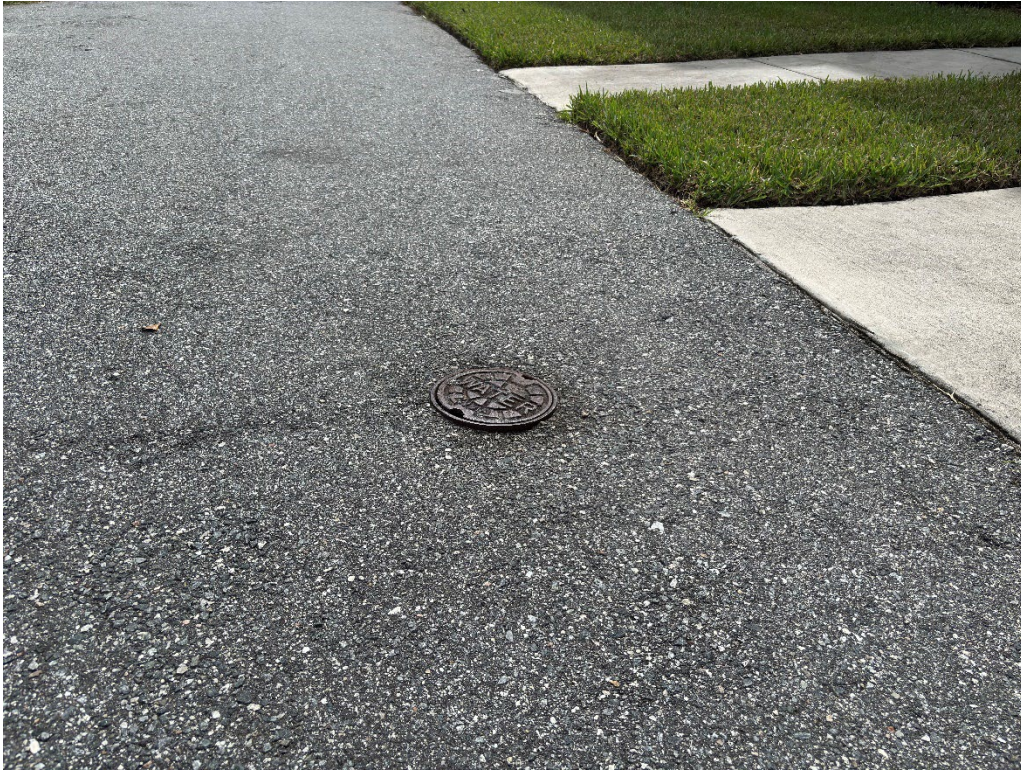
Photo 3 – Valve Cover Approximately 1 inch Reveal
