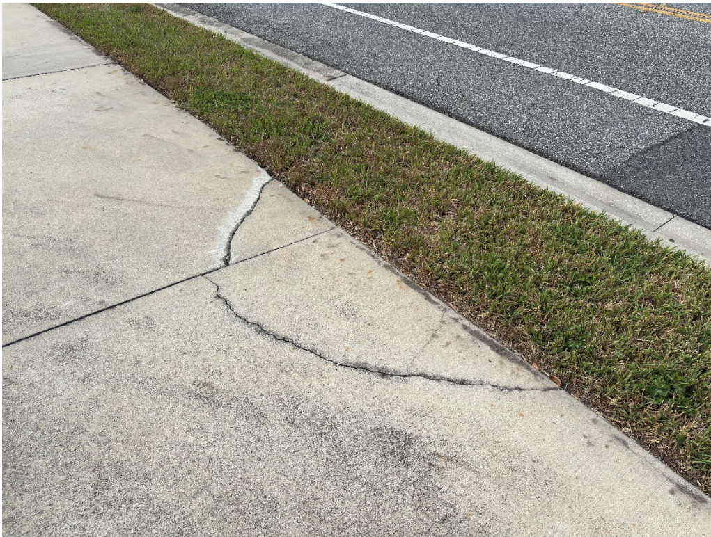
Photo 72 – Cracked Concrete and Base Failure
