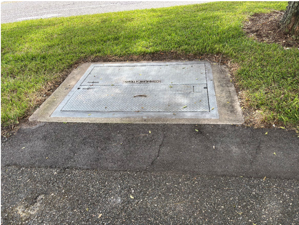
Photo 38 – Poor Quality Asphalt Patch
