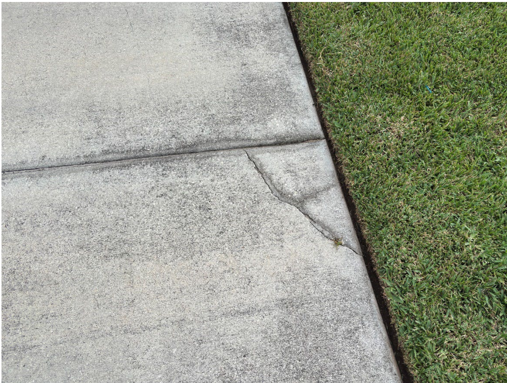
Photo 18 - Cracked Concrete and Base Failure
