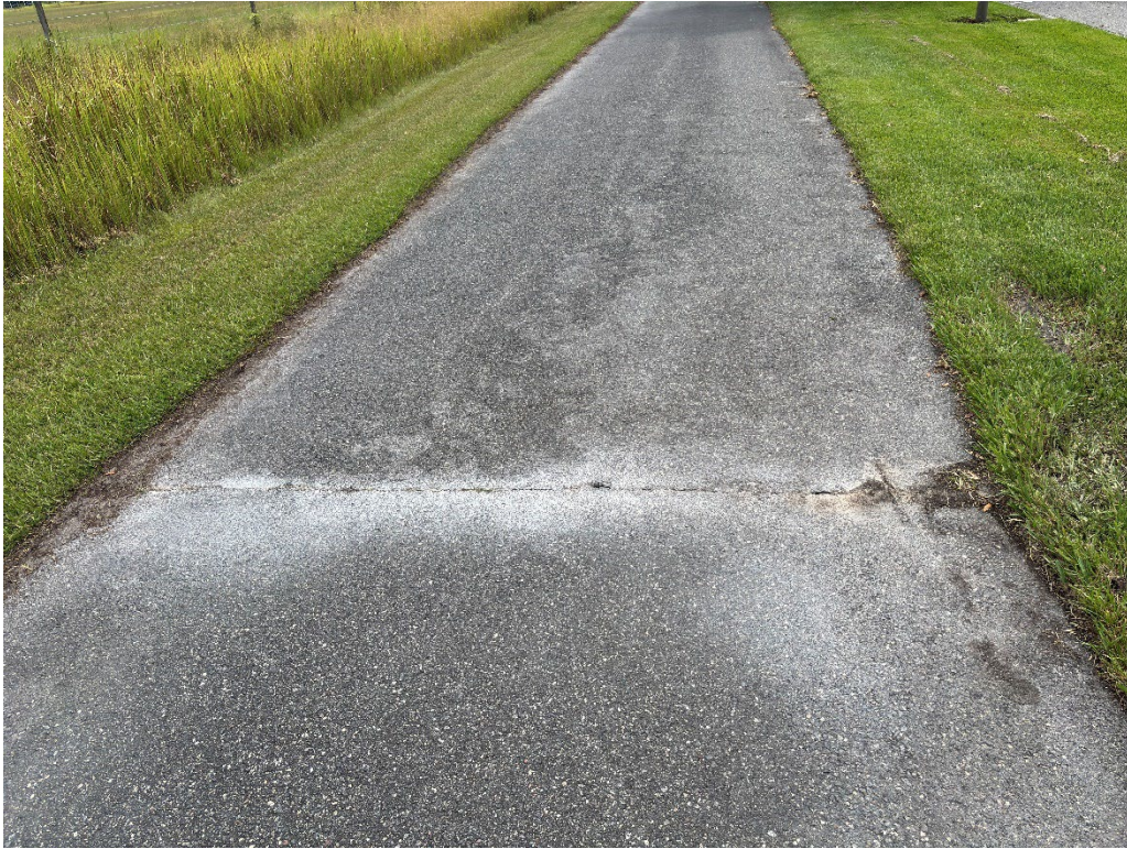
Photo 43 – Asphalt Raveling and Base Failure
