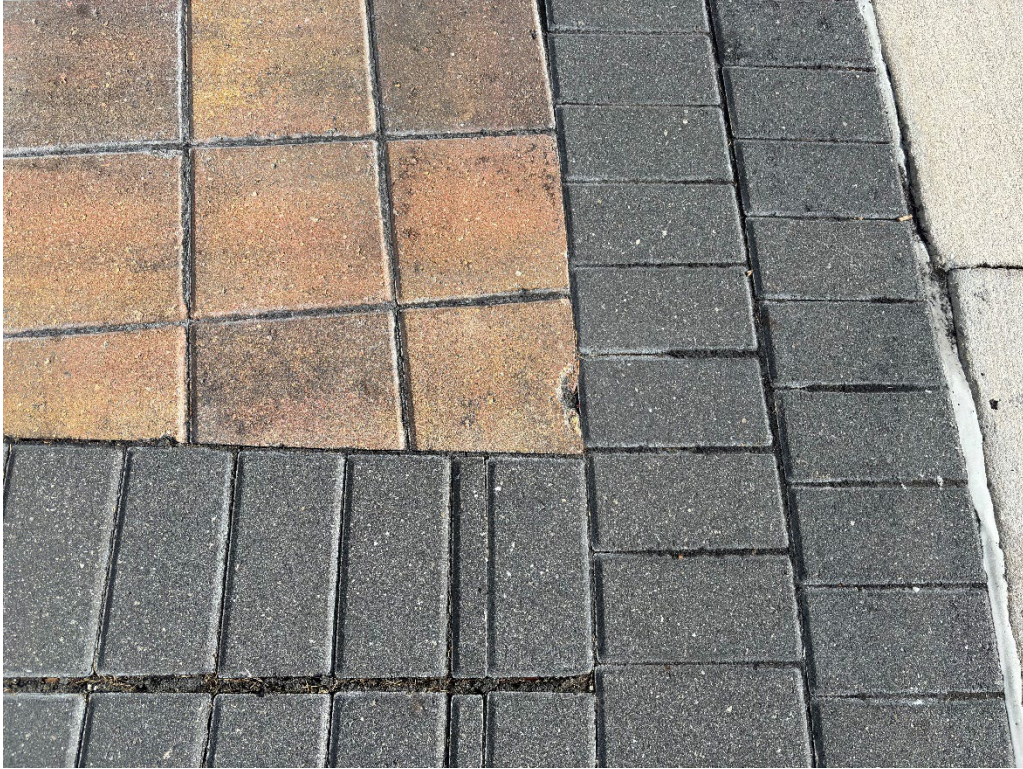
Photo 77 – Broken Concrete Pavers on Truck Apron
