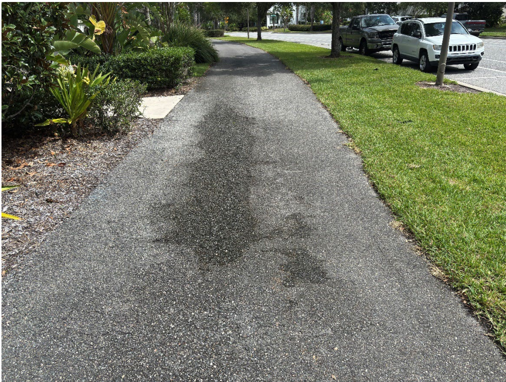
Photo 42 – Asphalt Raveling in Low Area
