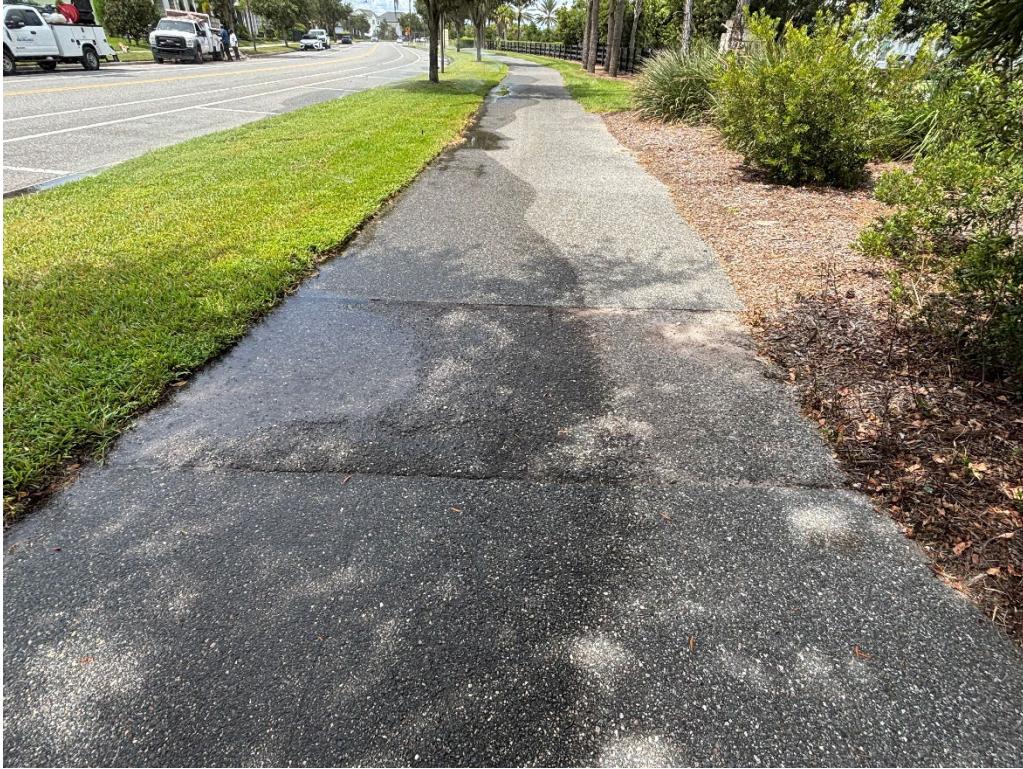
Photo 33 – Poor Quality Asphalt Patch
