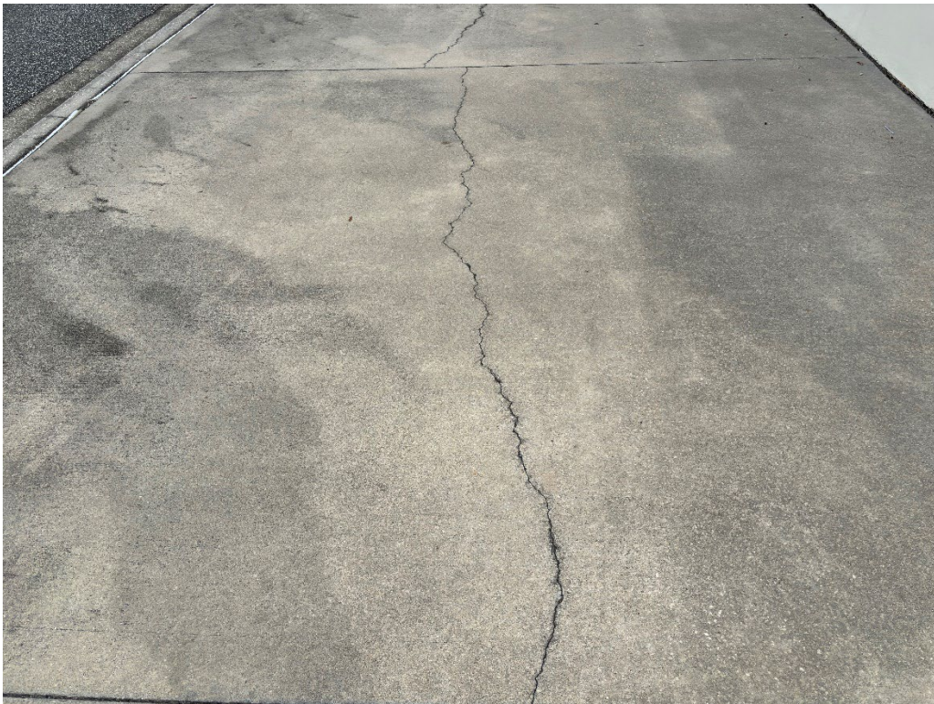
Photo 70 – Surficial Cracked Concrete
