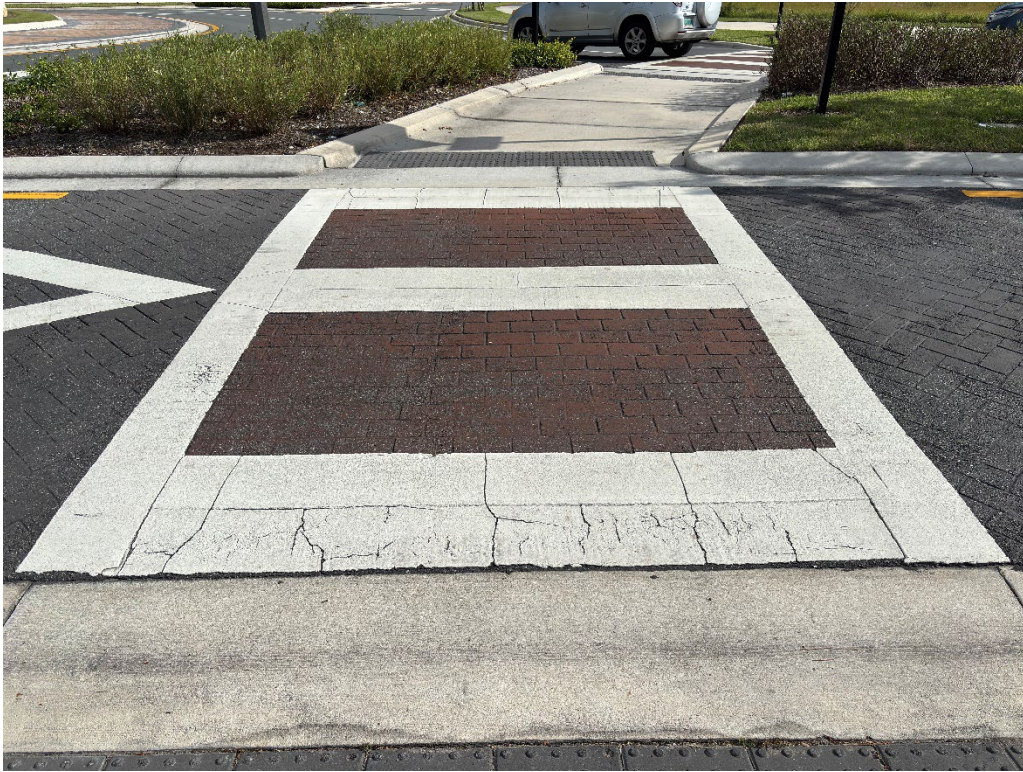
Photo 76 - Deteriorating Thermoplastic and Worn Crosswalk Coloration
