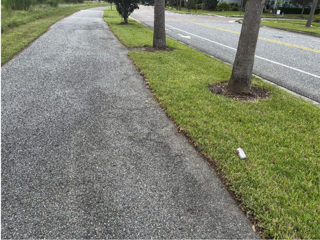
Photo 57 – Asphalt Raveling and Base Failure
