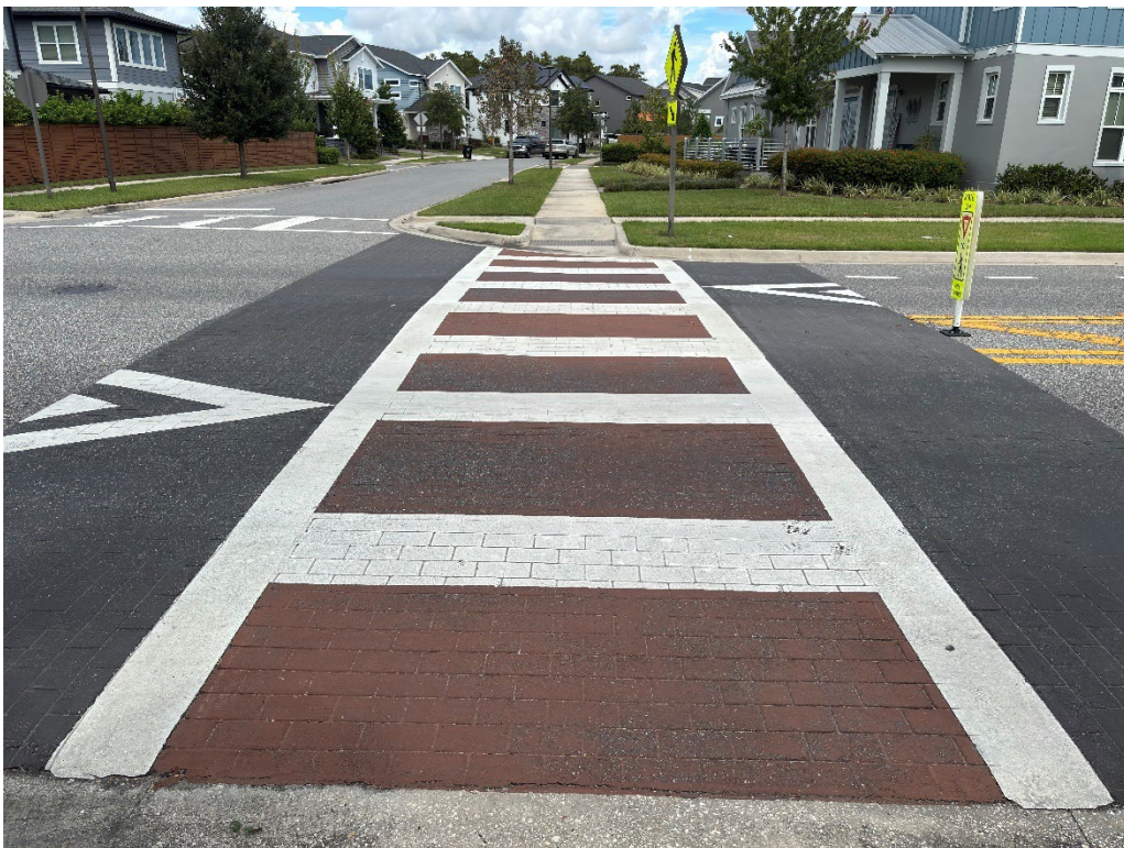
Photo 10 – Worn Crosswalk Coloration
