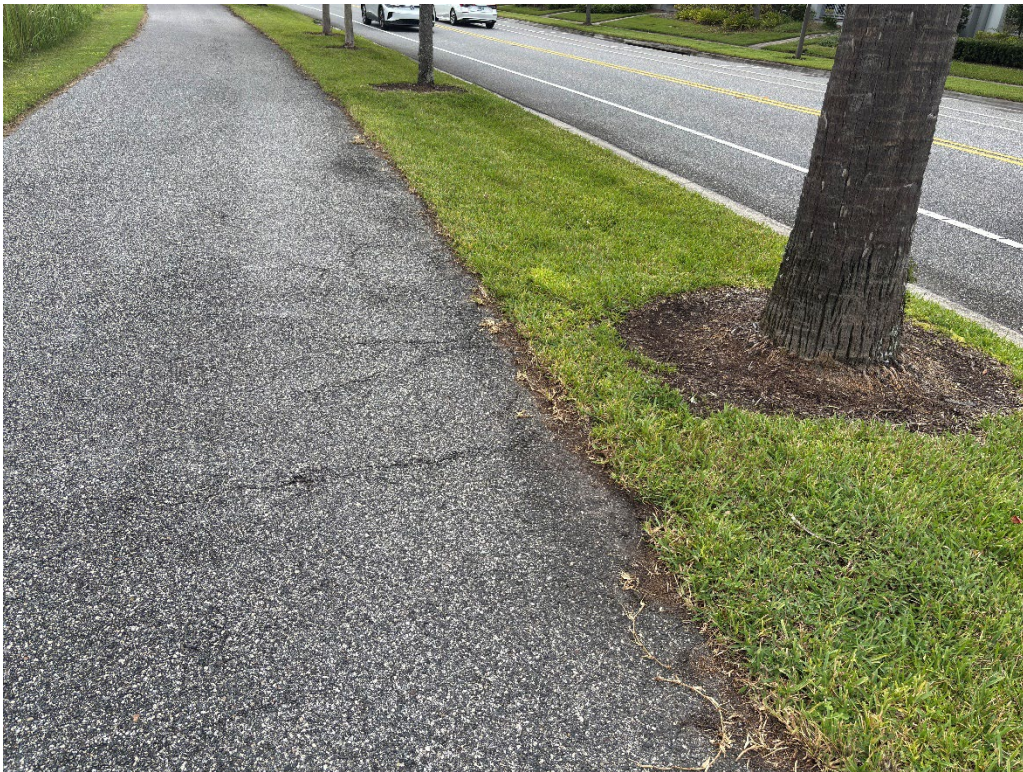
Photo 58 – Asphalt Raveling and Base Failure
