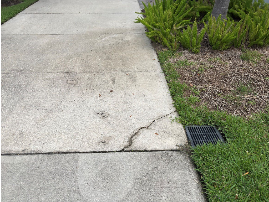
Photo 15 – Concrete Failure at Inlet
