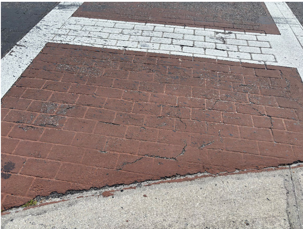
Photo 52 – Deteriorating Thermoplastic and Worn Crosswalk Coloration
