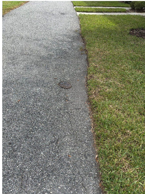
Photo 2 – Asphalt Pavement Edge Failure
