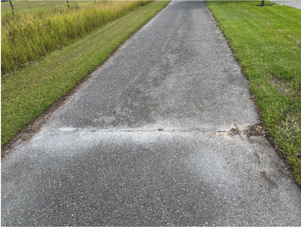
Photo 43 – Asphalt Raveling and Base Failure
