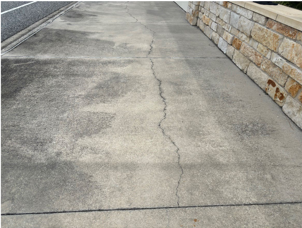
Photo 68 – Surficial Cracked Concrete
