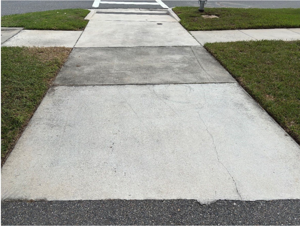
Photo 7 – Surficial Crack’s in Concrete
