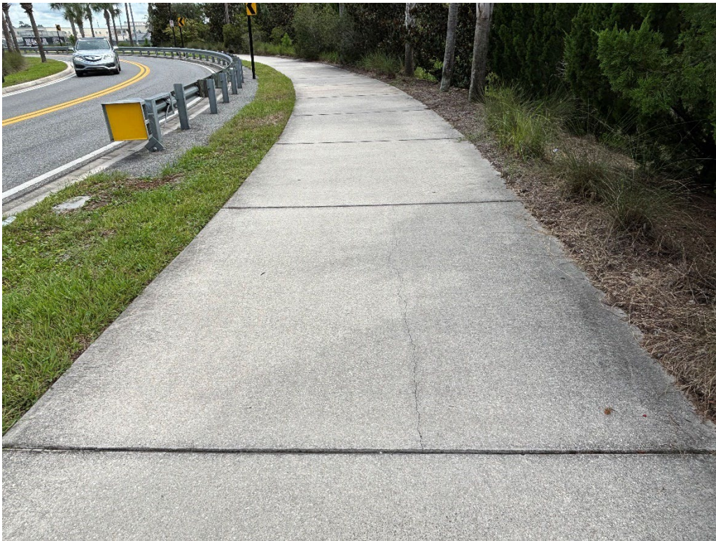
Photo 26 – Surficial Cracked Concrete
