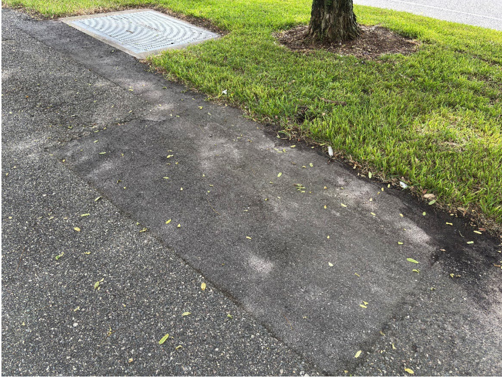
Photo 37 – Poor Quality Asphalt Patch
