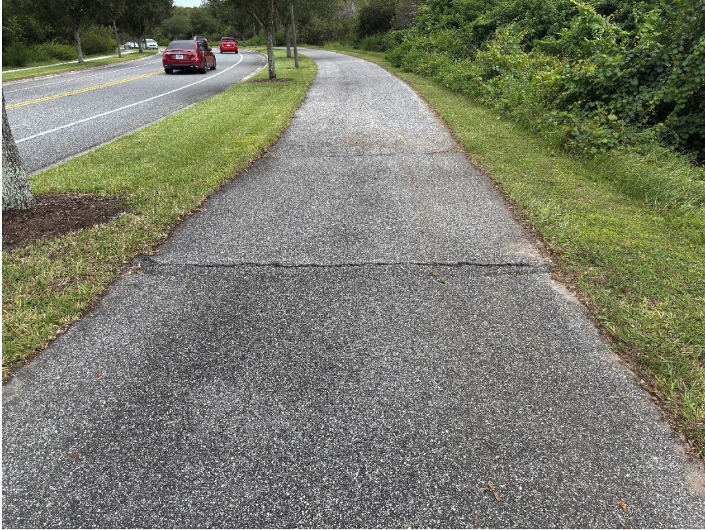
Photo 63 – Asphalt Patch Lifting
