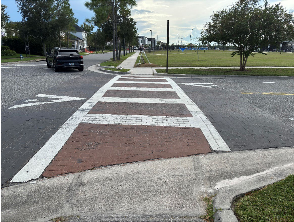
Photo 51 – Deteriorating Thermoplastic and Worn Crosswalk Coloration
