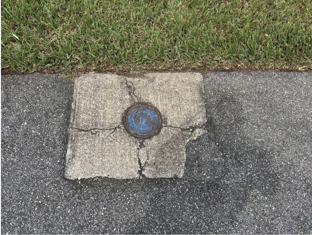
Photo 41 – Concrete Pad Valve Cover Cracked
