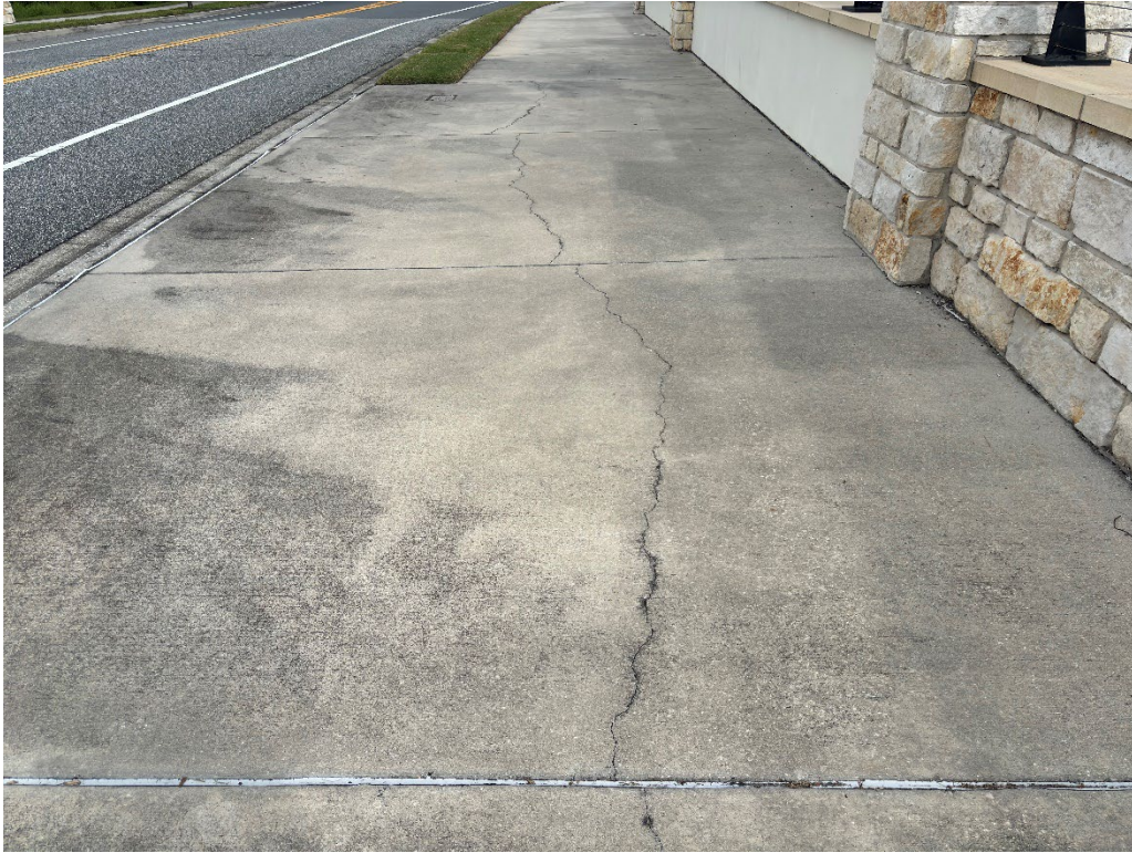
Photo 69 – Surficial Cracked Concrete
