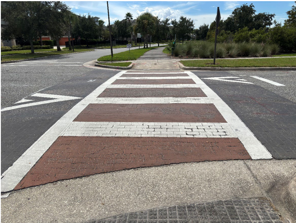
Photo 48 – Deteriorating Thermoplastic and Worn Crosswalk Coloration
