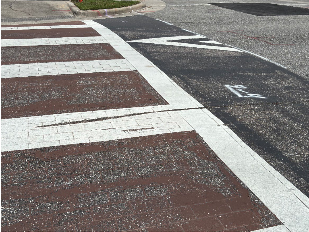
Photo 49 – Deteriorating Thermoplastic and Worn Crosswalk Coloration
