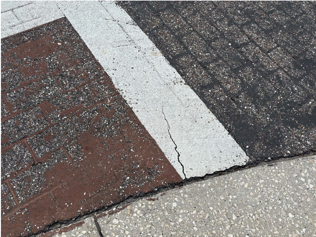
Photo 36 – Deteriorating Thermoplastic and Worn Crosswalk Coloration
