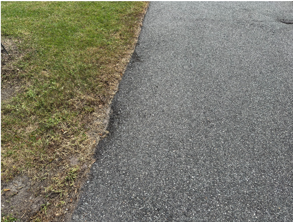
Photo 4 – Asphalt Pavement Edge Failure
