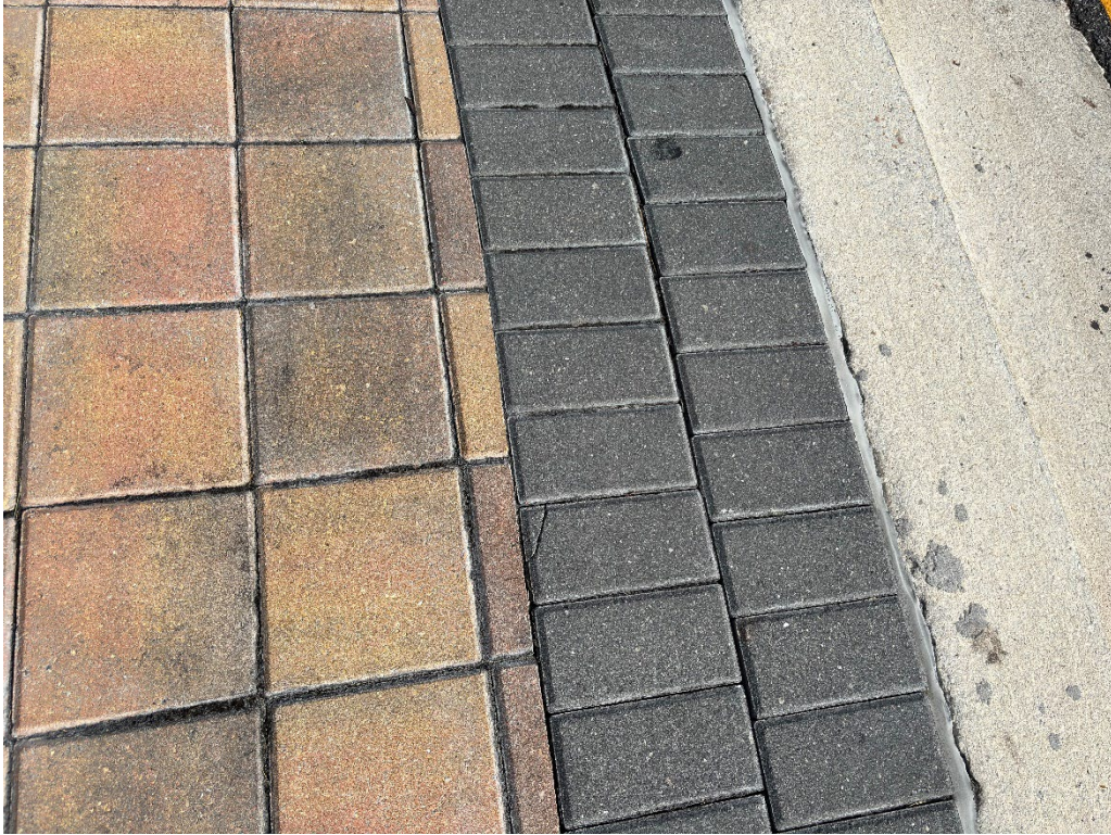
Photo 79 - Broken Concrete Pavers on Truck Apron
