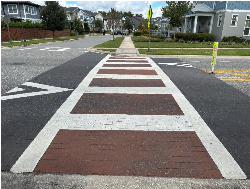
Photo 10 – Worn Crosswalk Coloration
