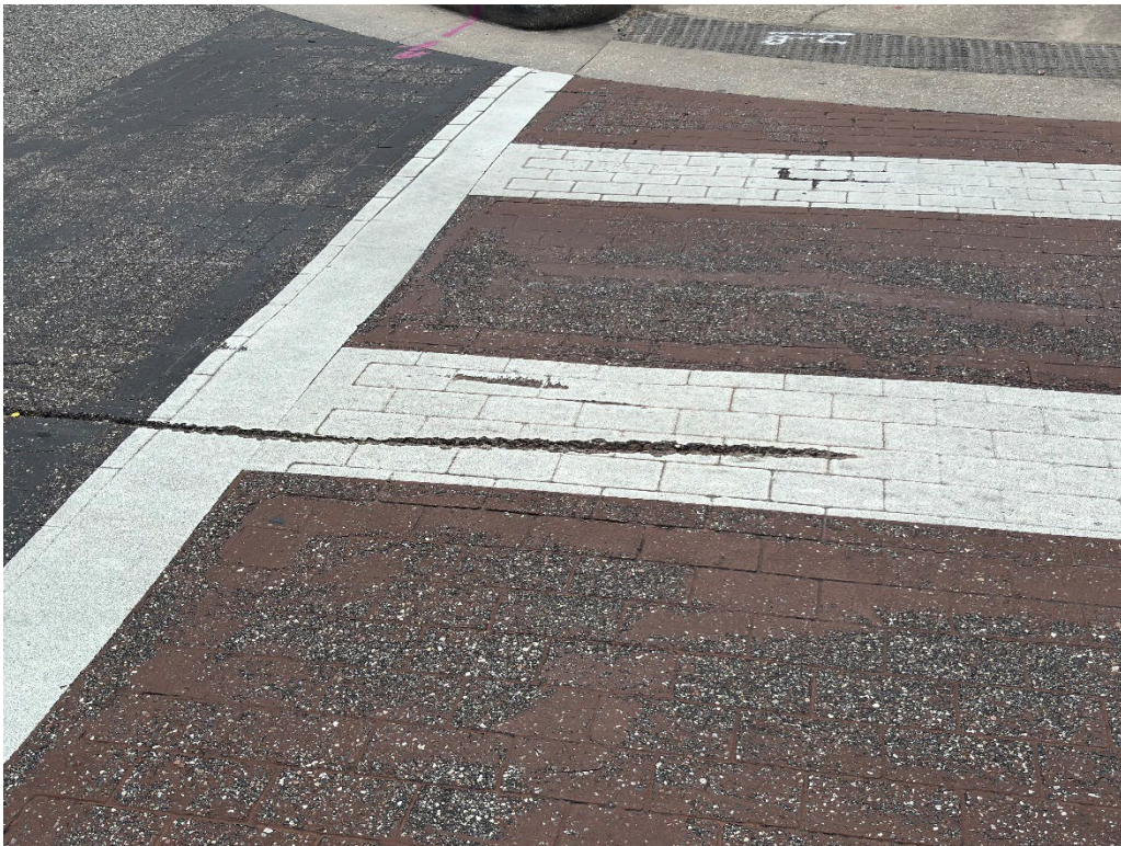
Photo 50 – Deteriorating Thermoplastic and Worn Crosswalk Coloration
