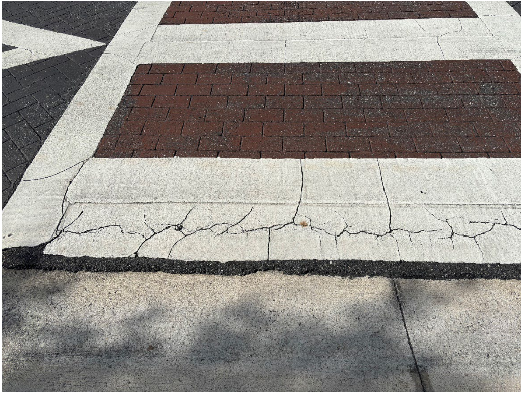
Photo 75 - Deteriorating Thermoplastic and Worn Crosswalk Coloration
