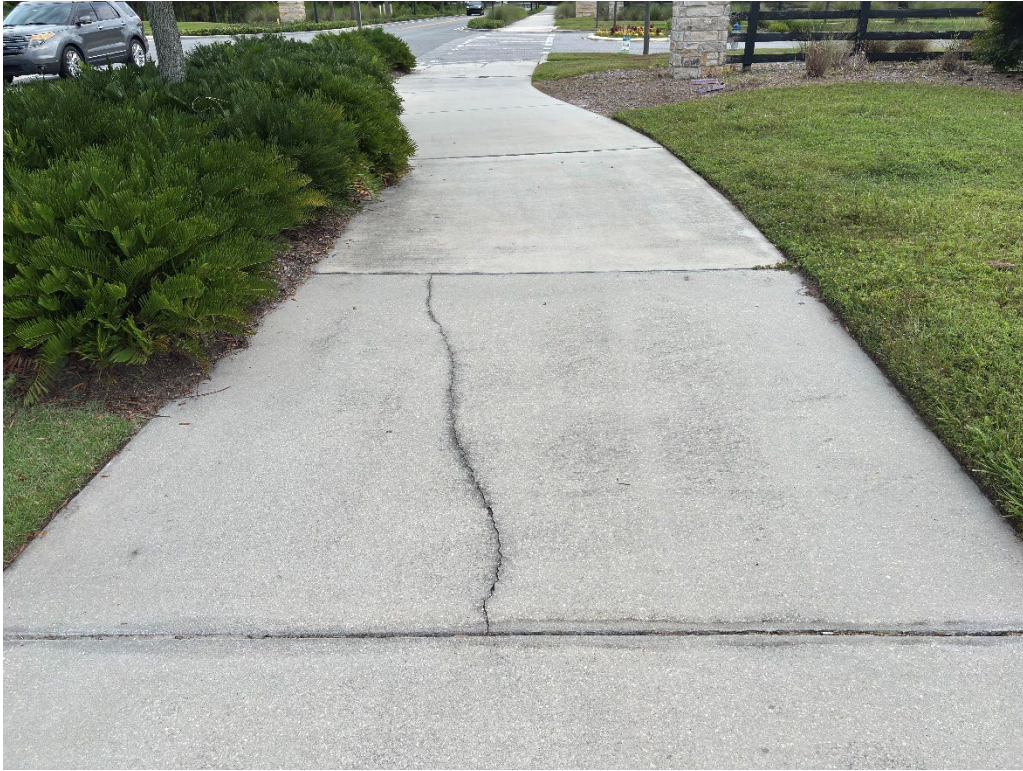
Photo 21 – Surficial Cracked Concrete
