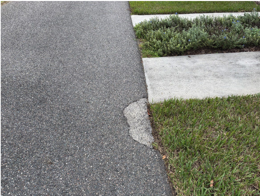
Photo 8 – Poor Asphalt Patch
