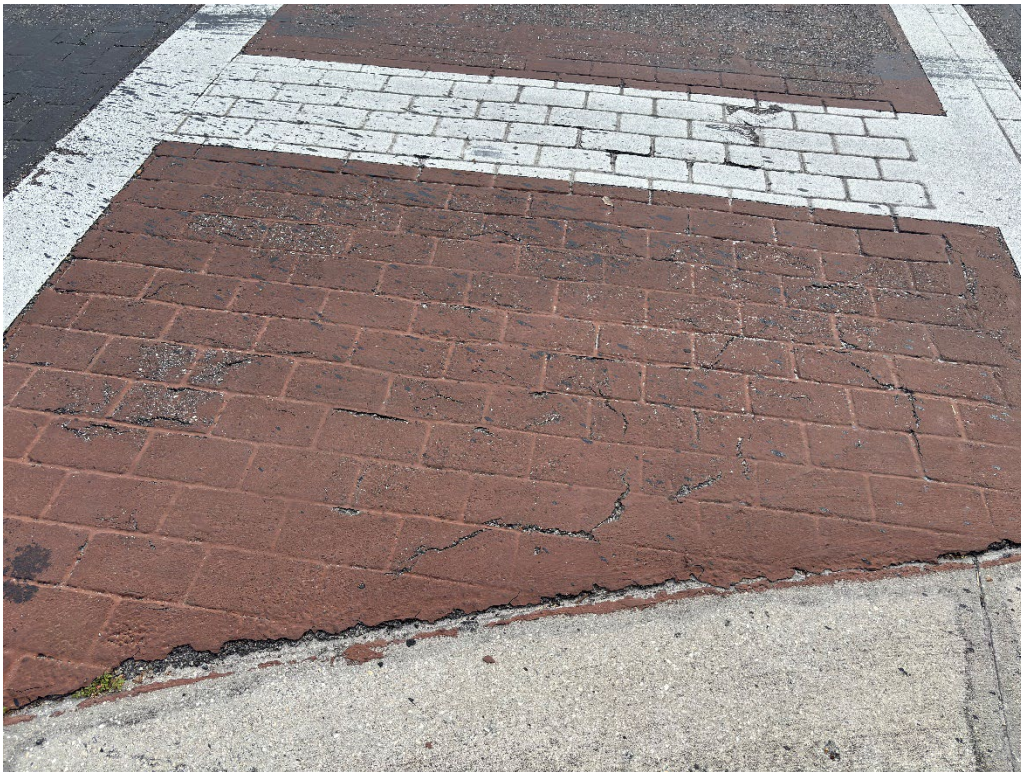
Photo 52 – Deteriorating Thermoplastic and Worn Crosswalk Coloration
