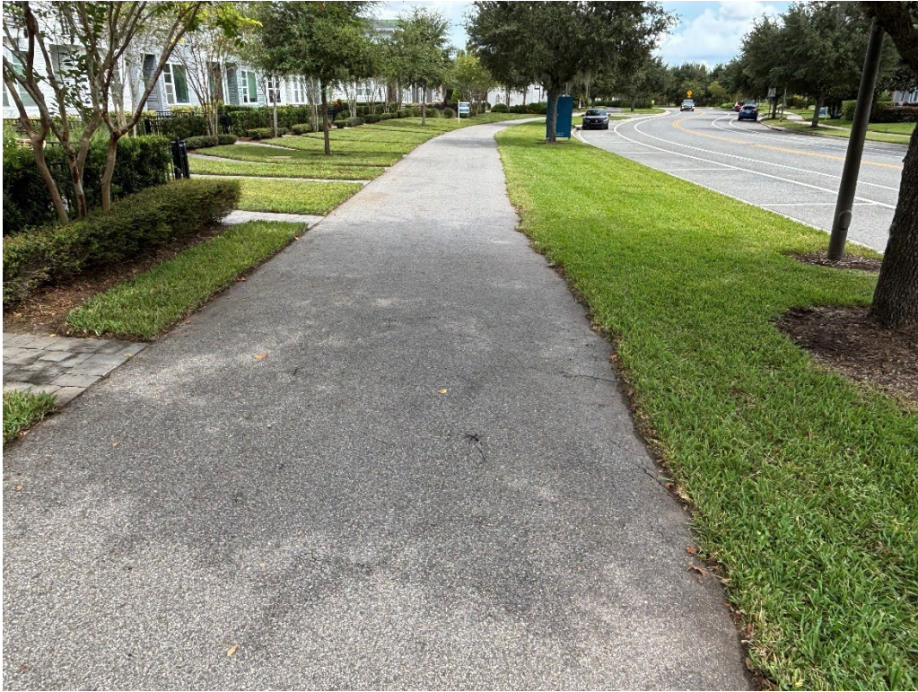
Photo 39 – Asphalt Edge Failure
