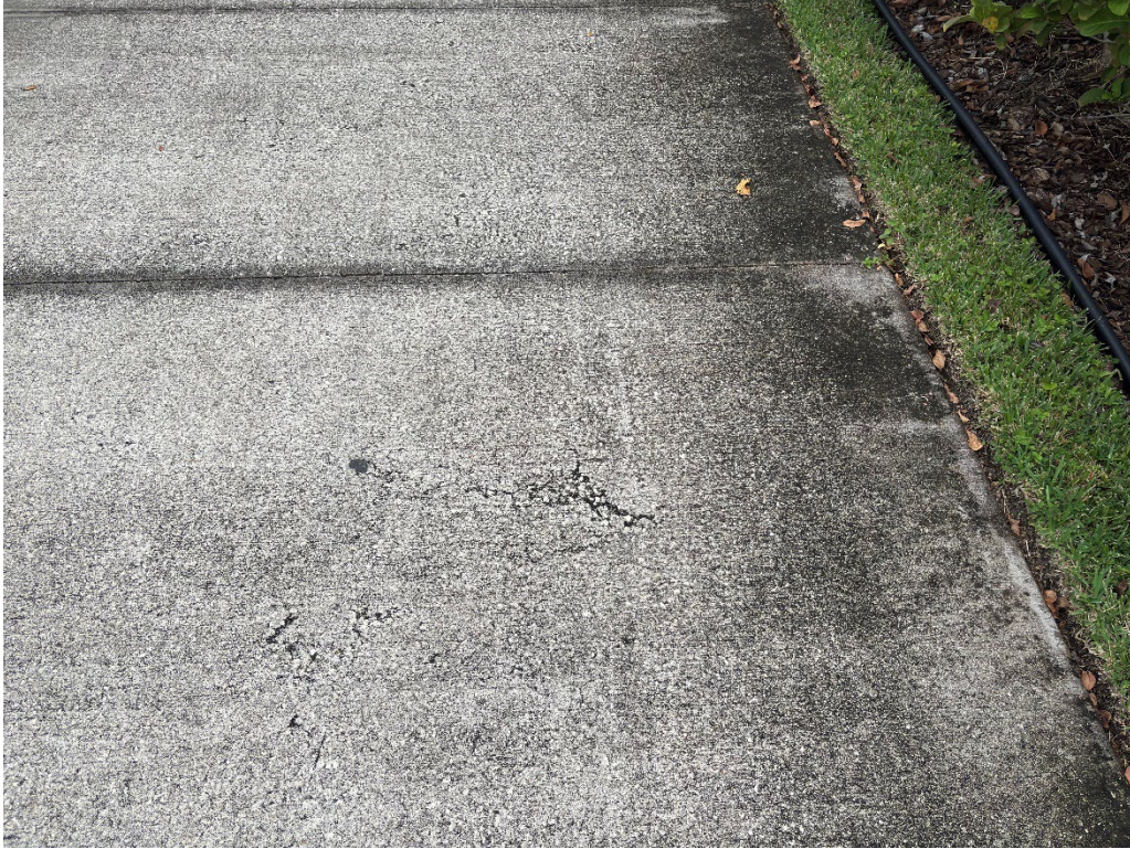
Photo 13 – Surficial Cracked Concrete
