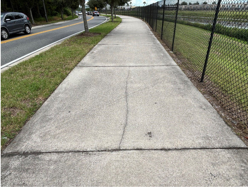
Photo 27 – Surficial Cracked Concrete
