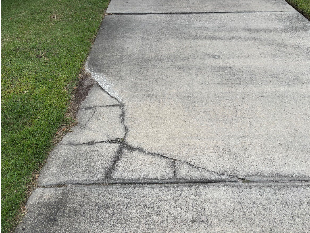
Photo 19 – Cracked Concrete and Base Failure
