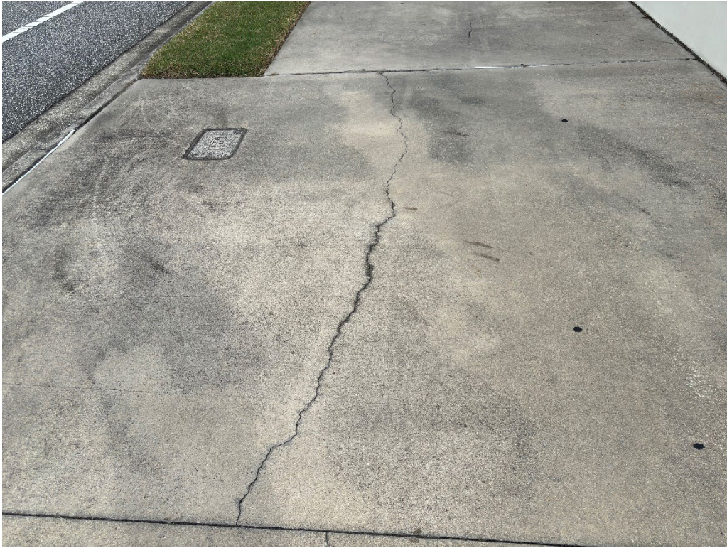
Photo 71 – Surficial Cracked Concrete
