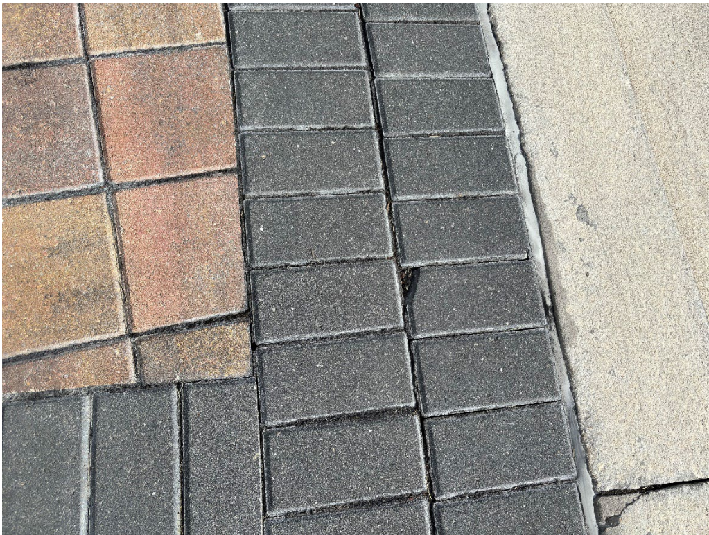
Photo 78 - Broken Concrete Pavers on Truck Apron
