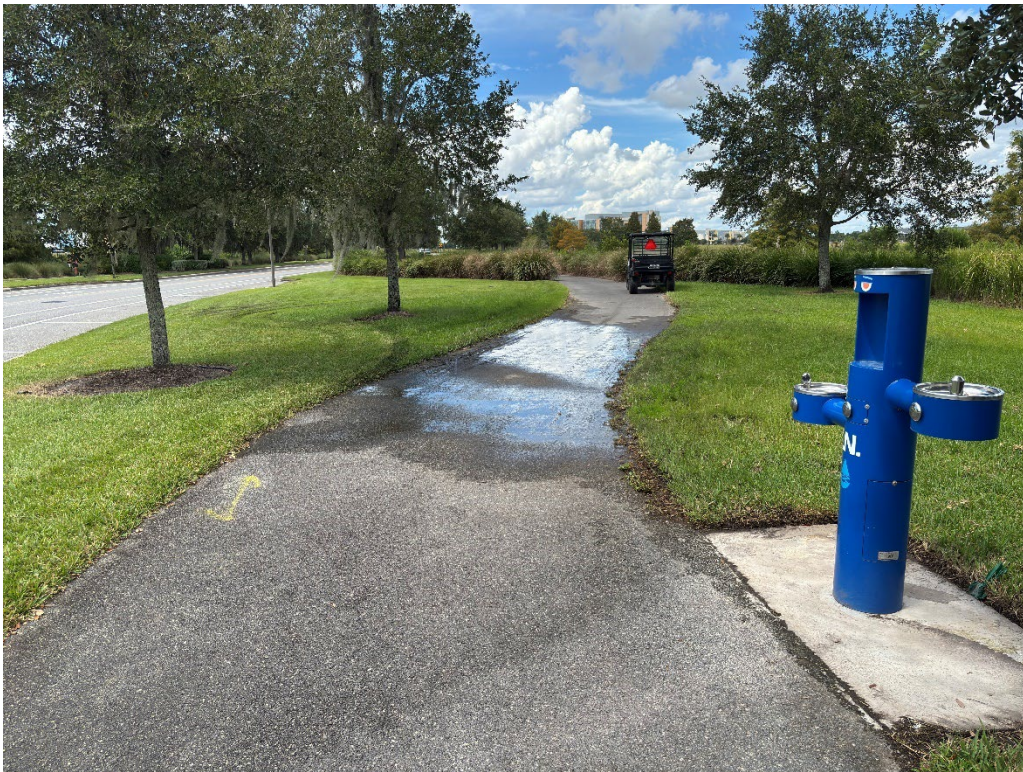
Photo 44 – Asphalt Raveling in Low Area
