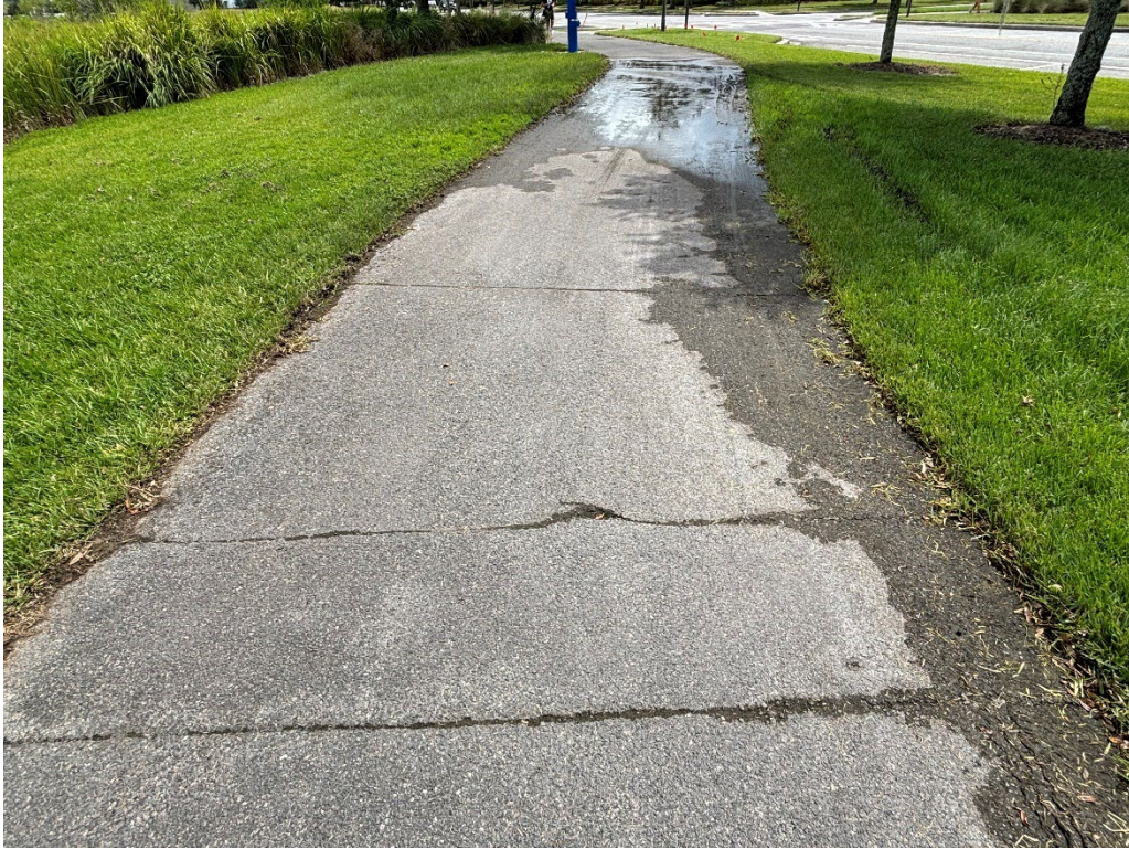
Photo 47 – Cracked Asphalt and Raveling in Low Area
