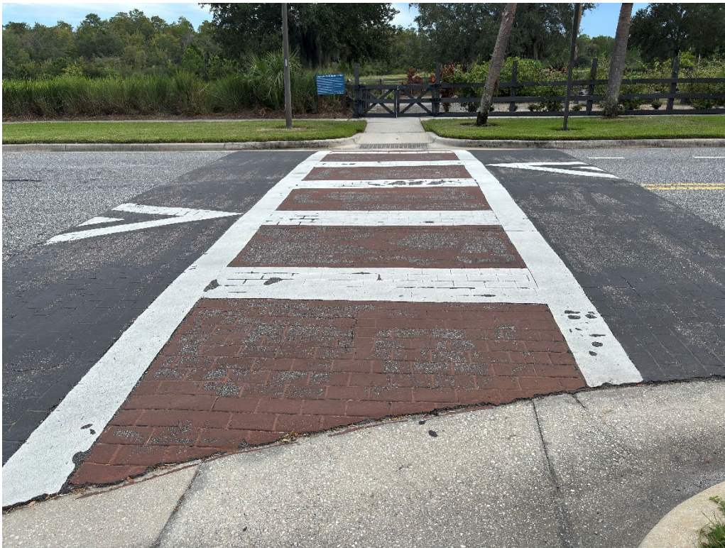
Photo 56 – Deteriorating Thermoplastic and Worn Crosswalk Coloration
