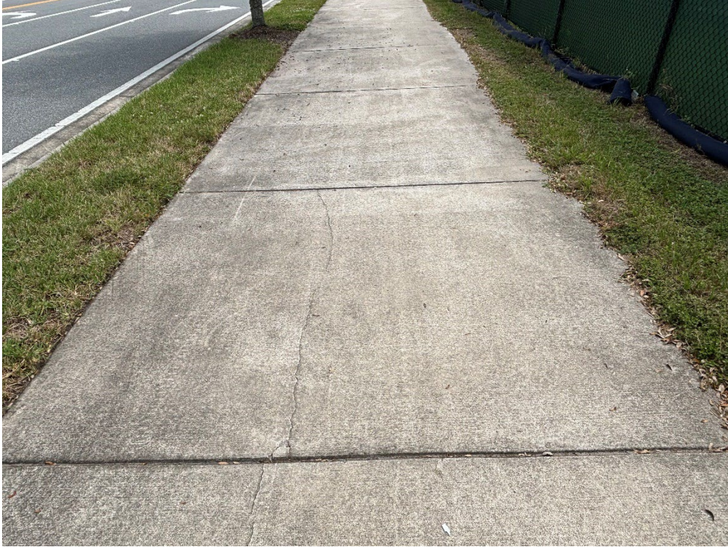
Photo 29 – Surficial Cracked Concrete
