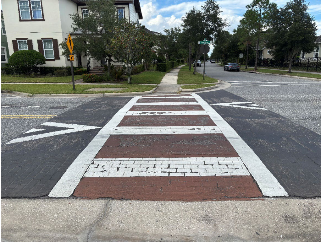
Photo 55 – Deteriorating Thermoplastic and Worn Crosswalk Coloration
