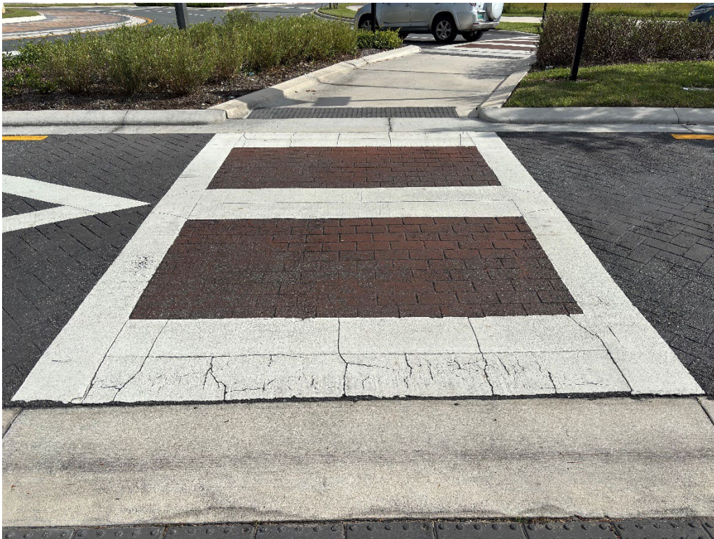
Photo 76 - Deteriorating Thermoplastic and Worn Crosswalk Coloration
