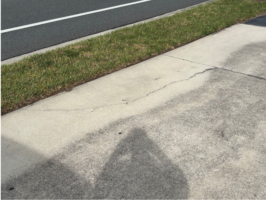
Photo 73 – Cracked Concrete Base Failure
