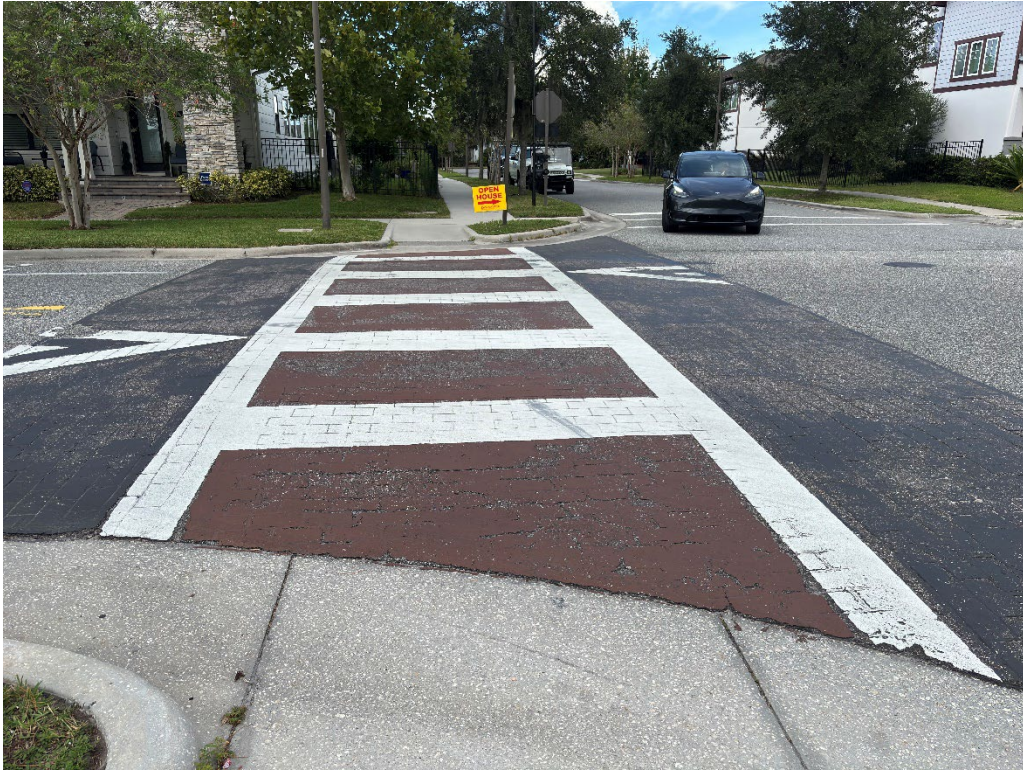
Photo 53 – Deteriorating Thermoplastic and Worn Crosswalk Coloration
