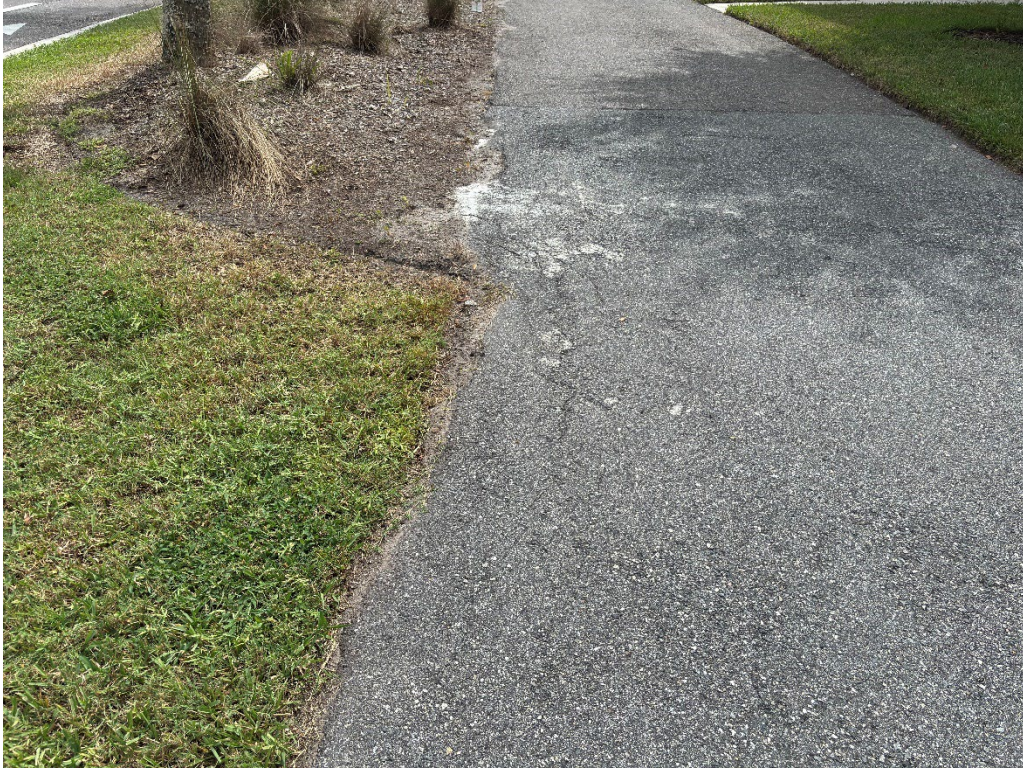
Photo 5 – Asphalt Pavement Edge Failure
