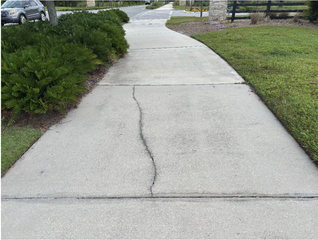
Photo 21 – Surficial Cracked Concrete
