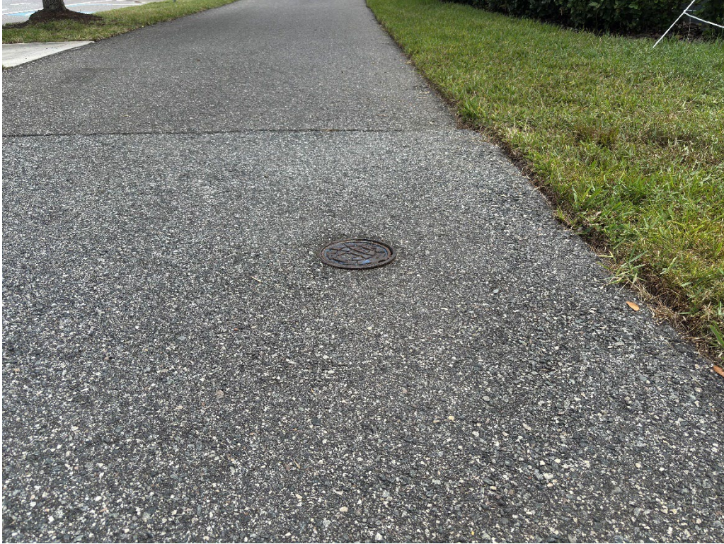
Photo 9 – Valve Cover Approximately 1/2-inch Reveal
