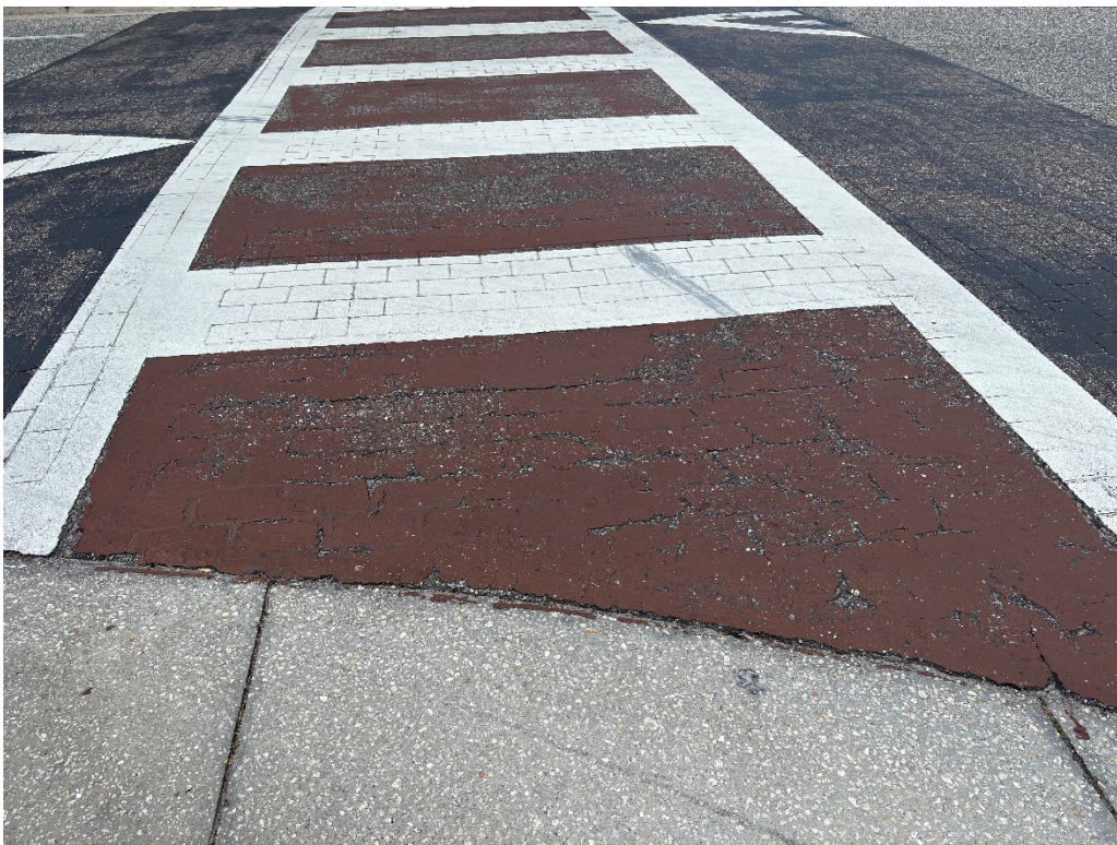
Photo 54 – Deteriorating Thermoplastic and Worn Crosswalk Coloration
