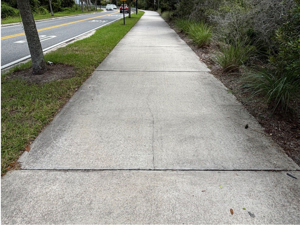
Photo 25 – Surficial Cracked Concrete
