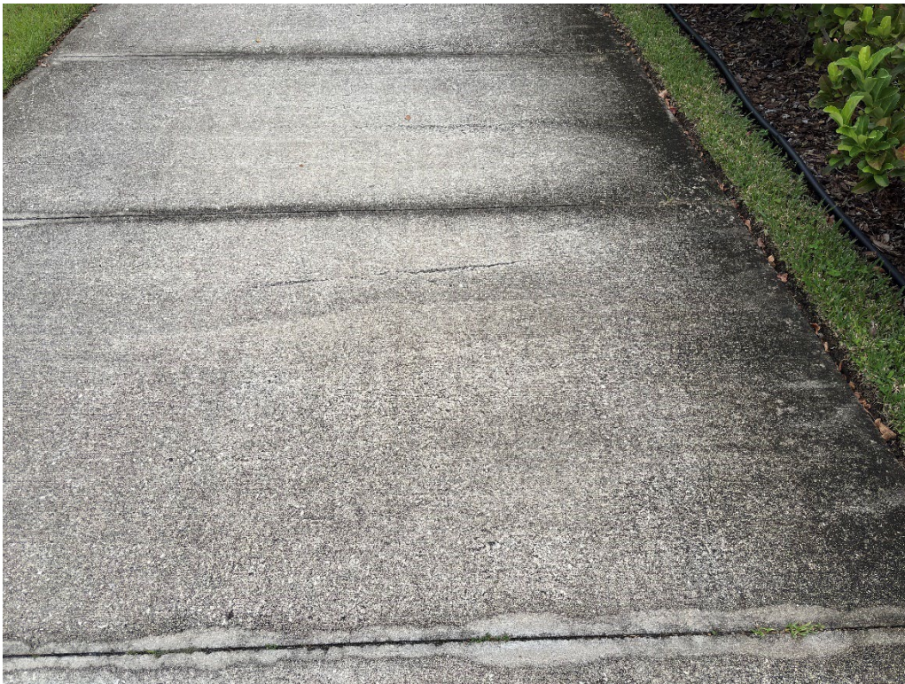
Photo 12 - Surficial Cracked Concrete
