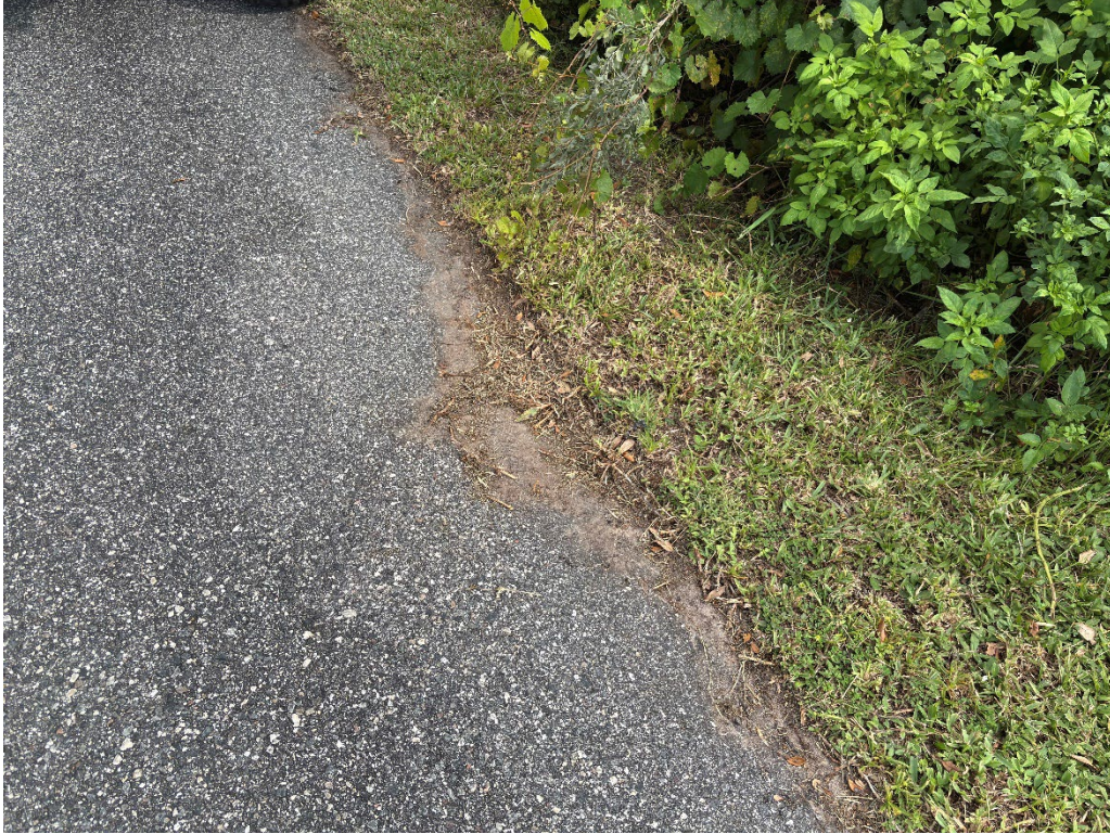
Photo 67 – Asphalt Edge Failure
