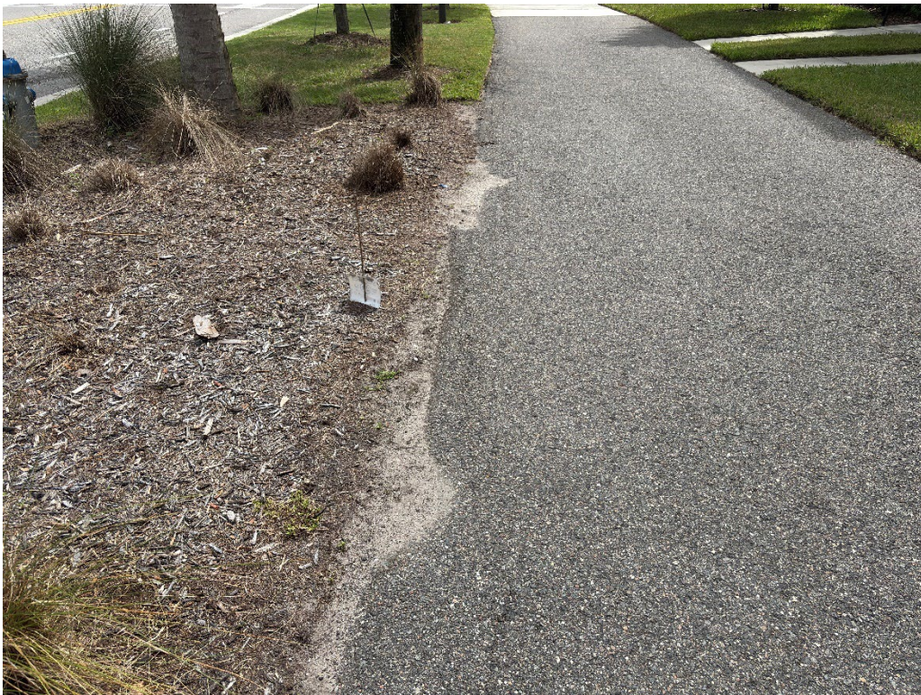
Photo 6 – Asphalt Pavement Edge Failure
