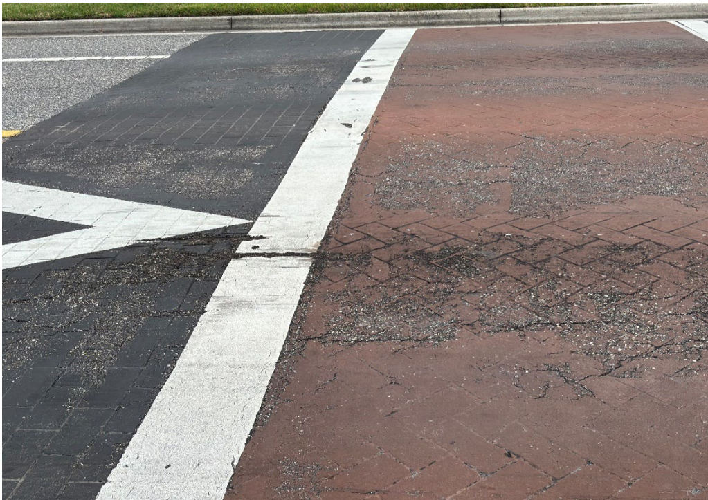
Photo 62 – Deteriorating Thermoplastic, Worn Crosswalk Coloration, and Asphalt Speed Table Deformation
