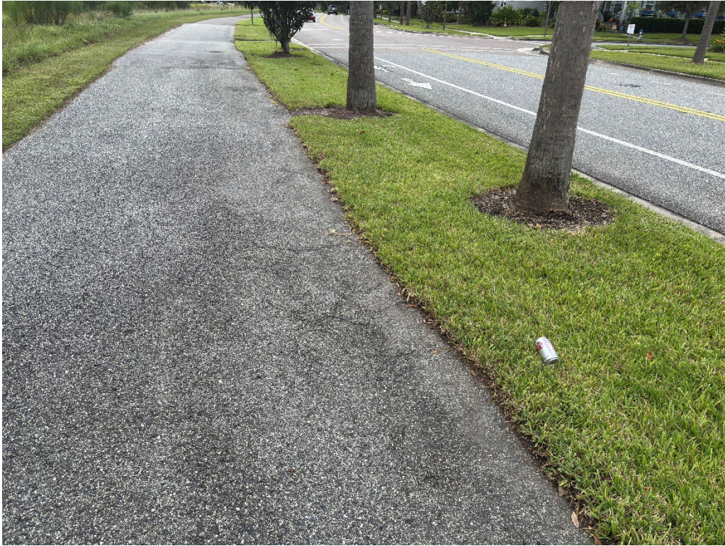
Photo 57 – Asphalt Raveling and Base Failure
