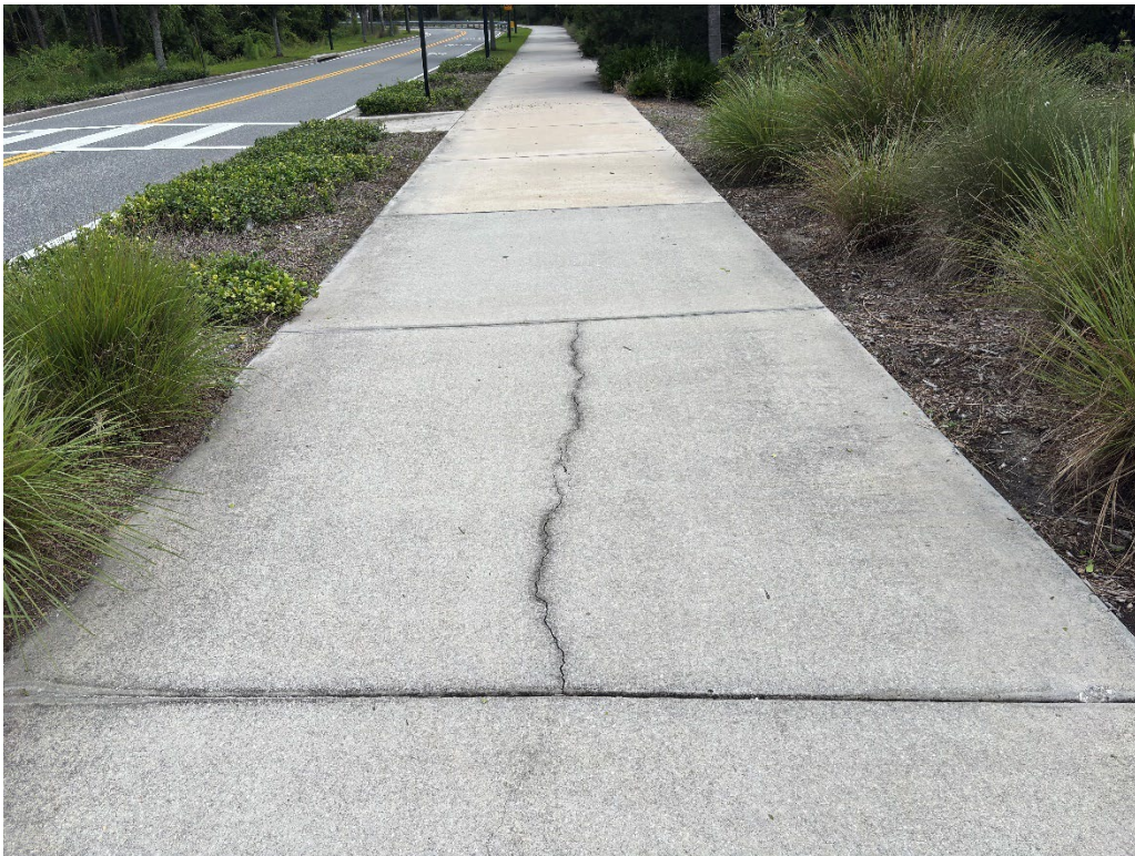
Photo 24 – Surficial Cracked Concrete
