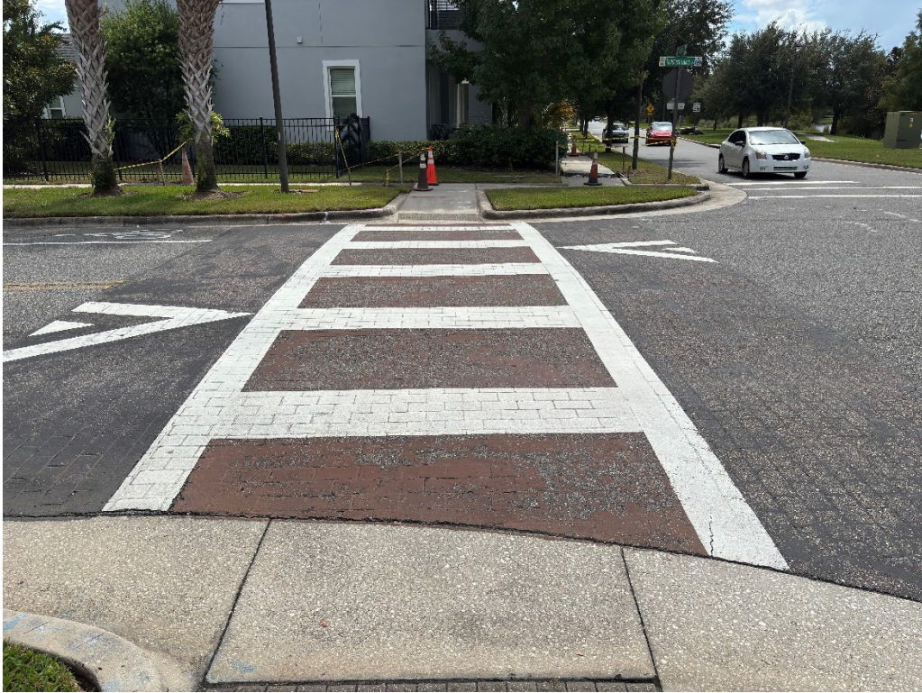
Photo 35 - Deteriorating Thermoplastic and Worn Crosswalk Coloration
