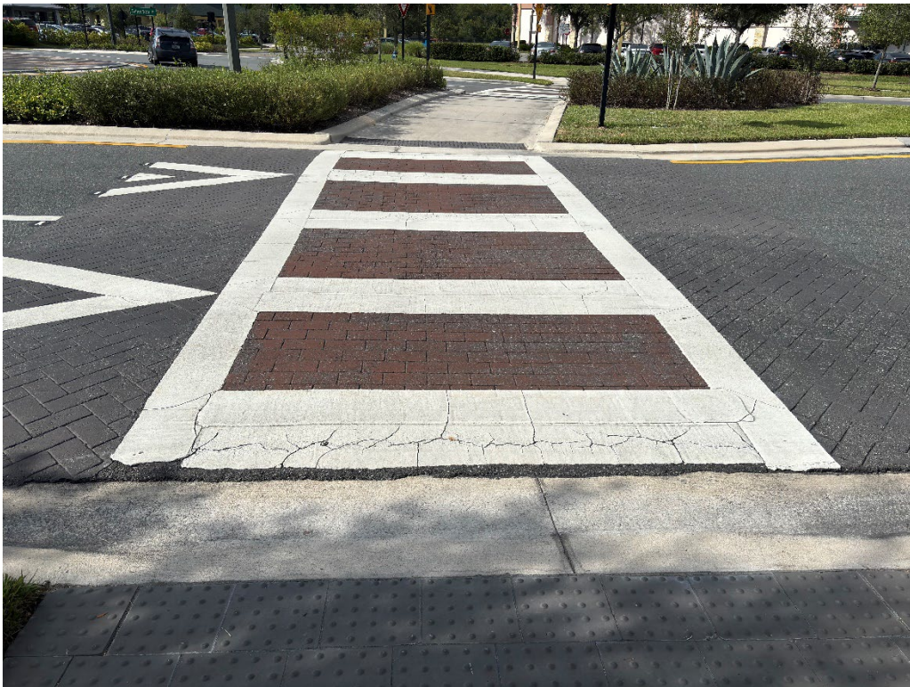
Photo 74 – Deteriorating Thermoplastic and Worn Crosswalk Coloration
