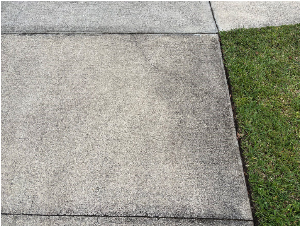
Photo 14 – Cracked Concrete and Base Failure
