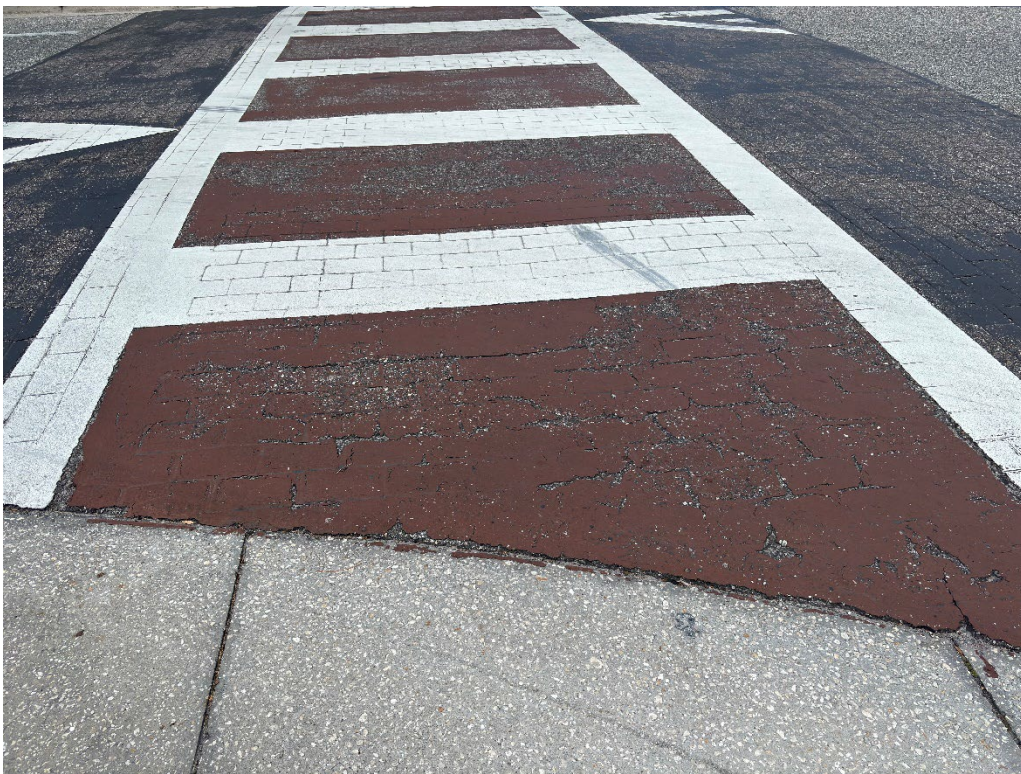
Photo 54 – Deteriorating Thermoplastic and Worn Crosswalk Coloration
