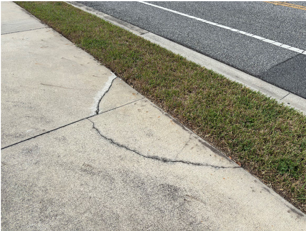
Photo 72 – Cracked Concrete and Base Failure
