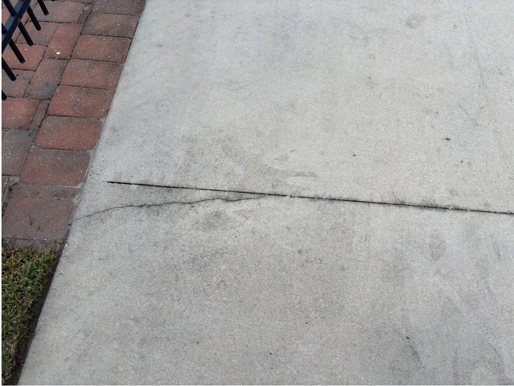
Photo 17 – Surficial Cracked Concrete
