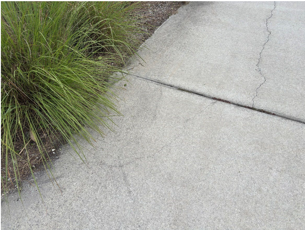
Photo 22 – Surficial Cracked Concrete
