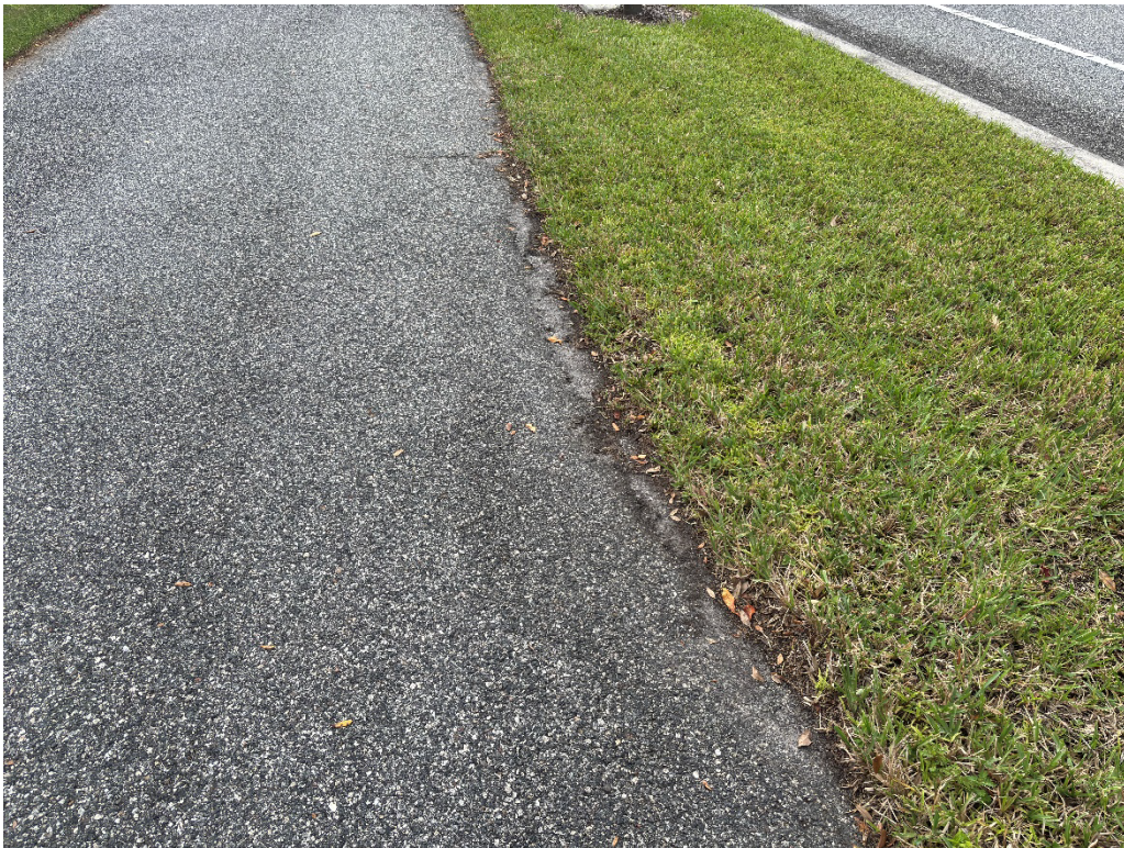
Photo 60 – Asphalt Pavement Edge Failure
