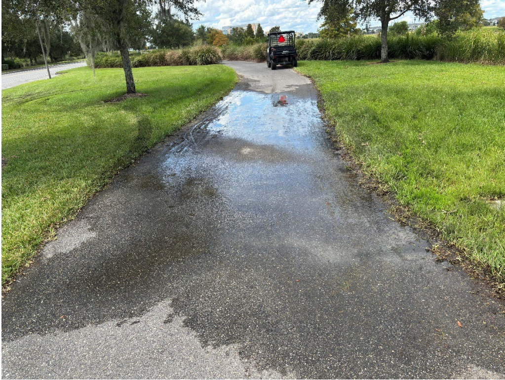
Photo 45 – Asphalt Raveling in Low Area
