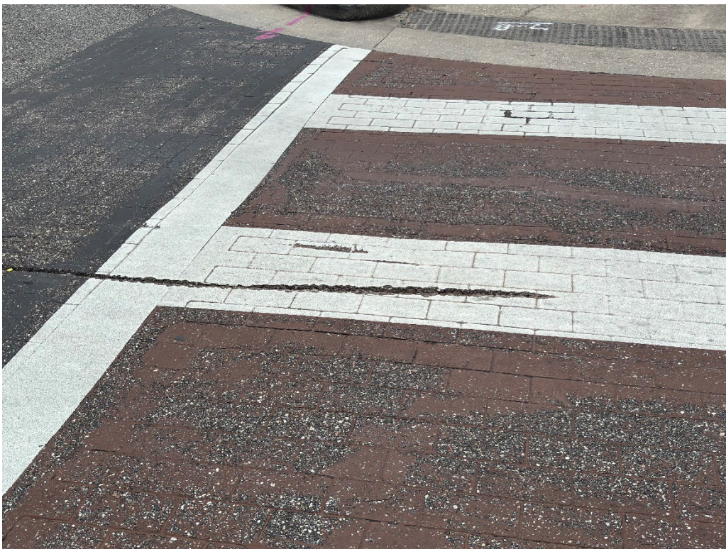
Photo 50 – Deteriorating Thermoplastic and Worn Crosswalk Coloration
