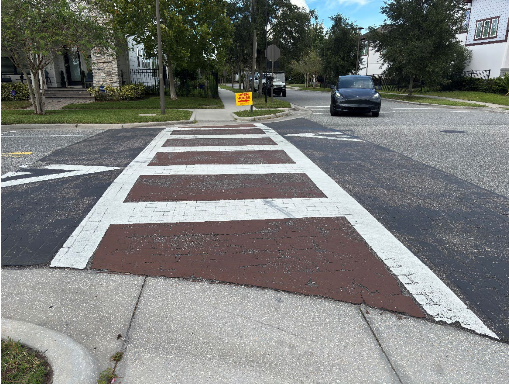
Photo 53 – Deteriorating Thermoplastic and Worn Crosswalk Coloration
