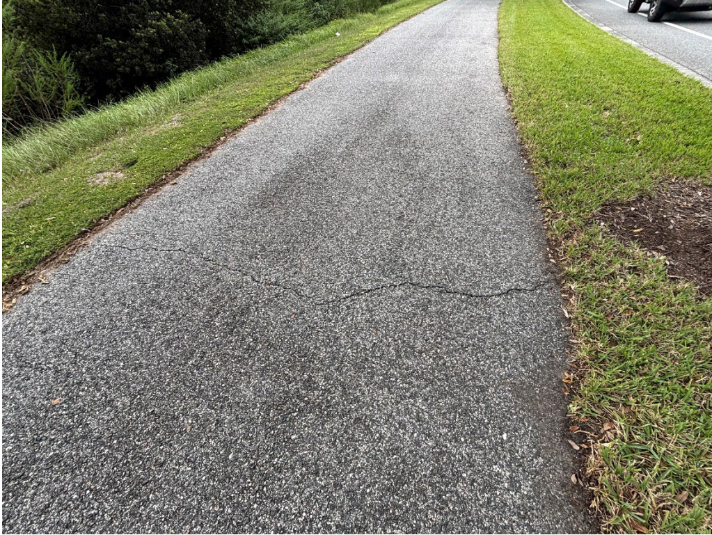
Photo 65 – Cracked Asphalt from Side to Side
