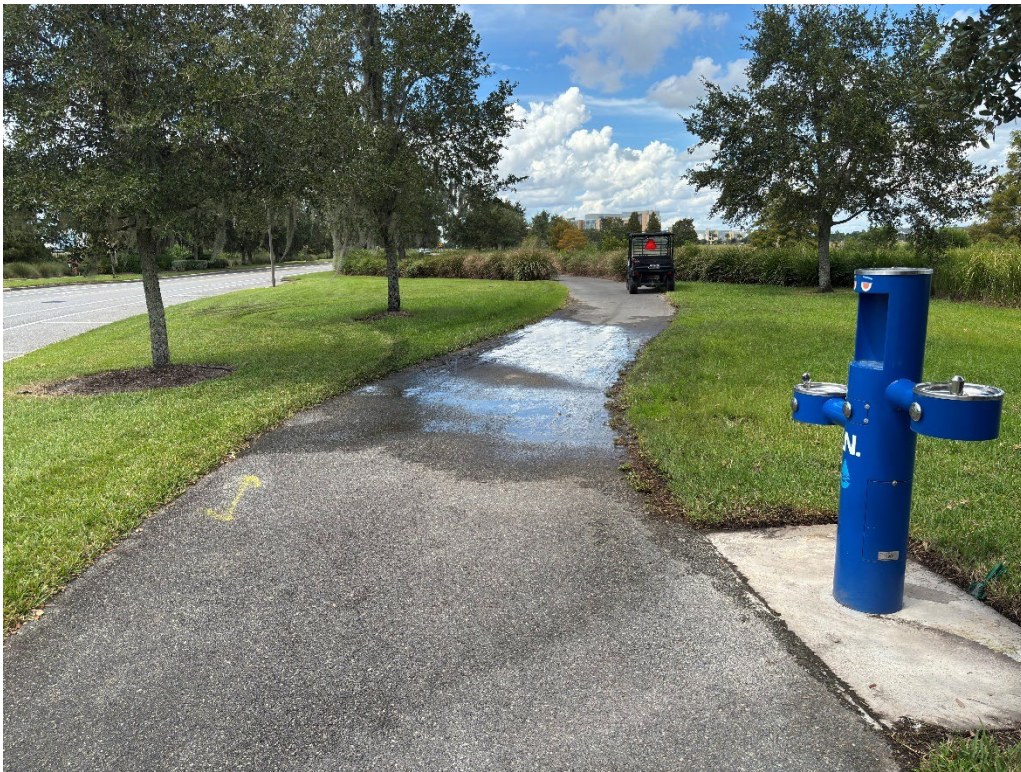
Photo 44 – Asphalt Raveling in Low Area
