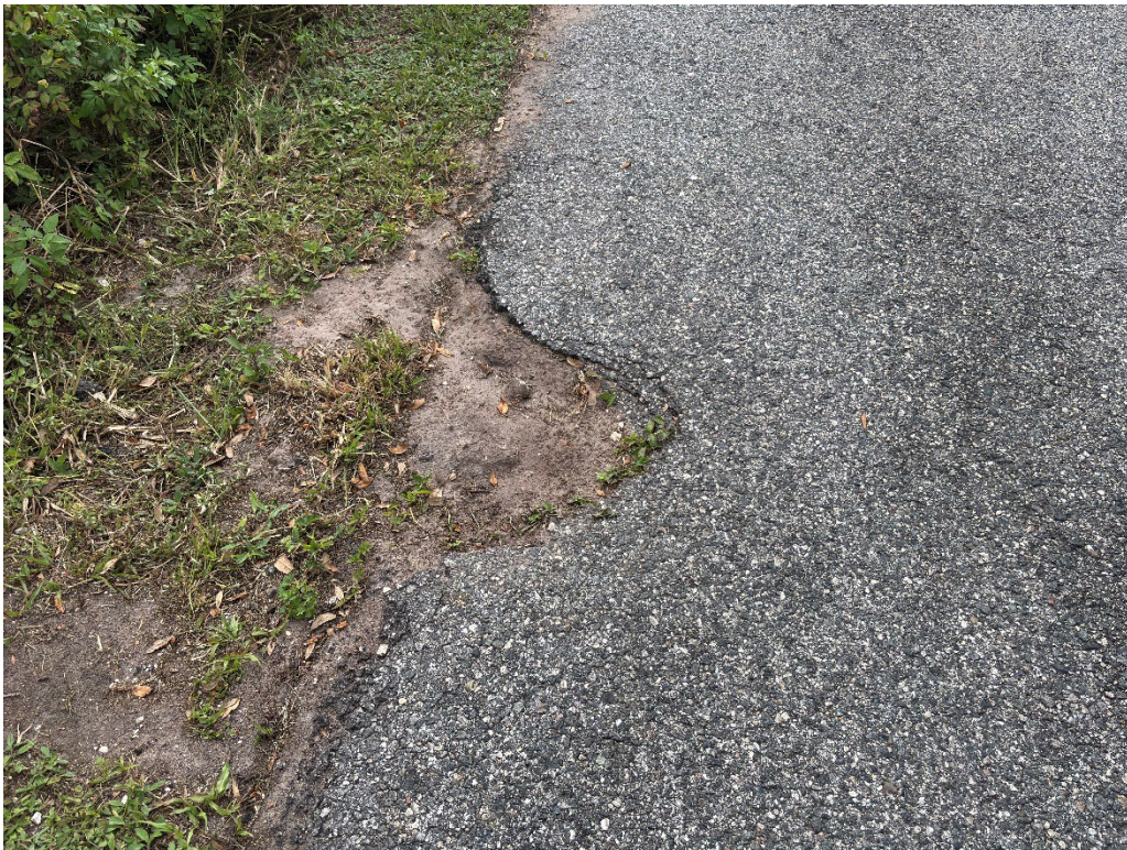
Photo 66 – Asphalt Edge Failure
