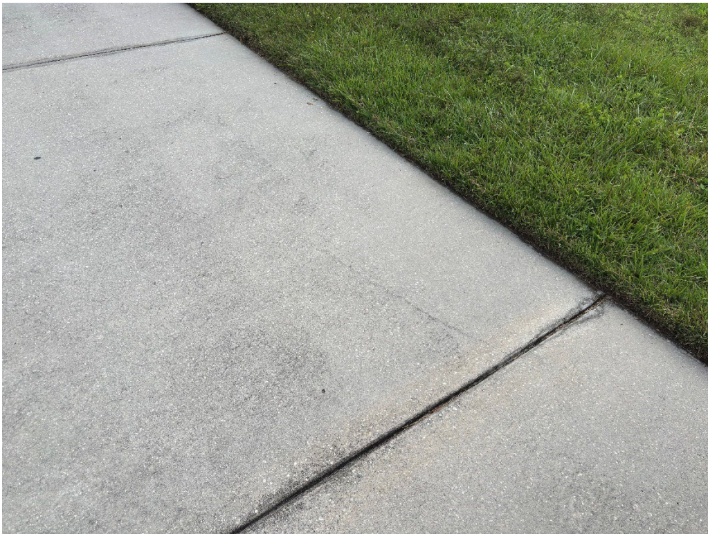
Photo 20 – Surficial Cracked Concrete
