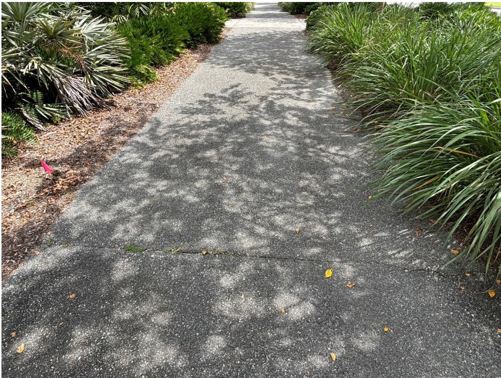
Photo 32 – Cracked Asphalt from Side to Side
